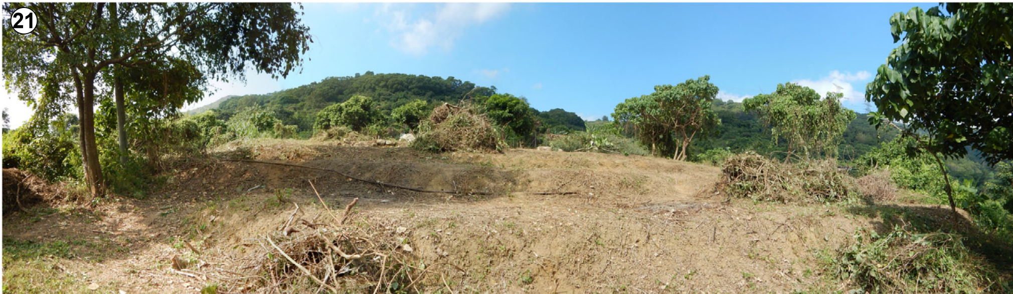
B 區 - 正進行地盤整理工程(在分區計劃大綱圖刊憲時觀察到的場地狀況) AREA B - SITE PREPARATION WORK IN PROGRESS (SITE CONDITION OBSERVED AT THE TIME OF GAZETTAL OF OUTLINE ZONING PLAN)
