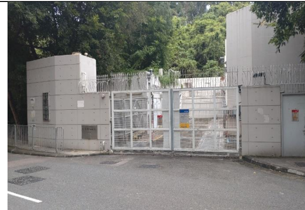
Photo 8: Tin Shui Wai Light Rail Substation
