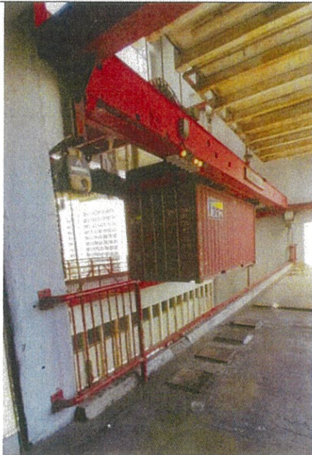
Fig 3. Hoisting machine carrying raw materials containers to the production line from G/F to upper floors
