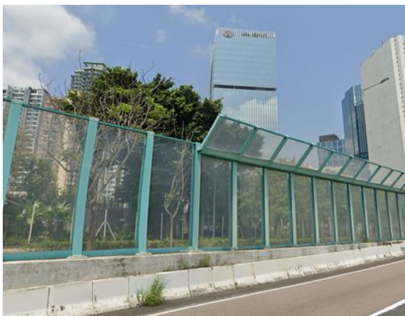
Noise barrier with fewer/without sub-frame at Island Eastern Corridor near Taikoo, Hong Kong
