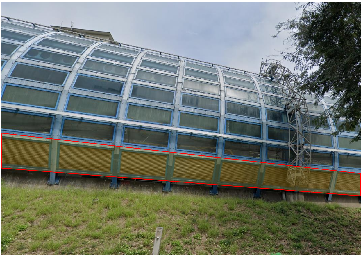
Figure 2.8.7 Example of Acoustic Louvres in Noise Enclosures, on Wong Chu Road, Tuen Mun
