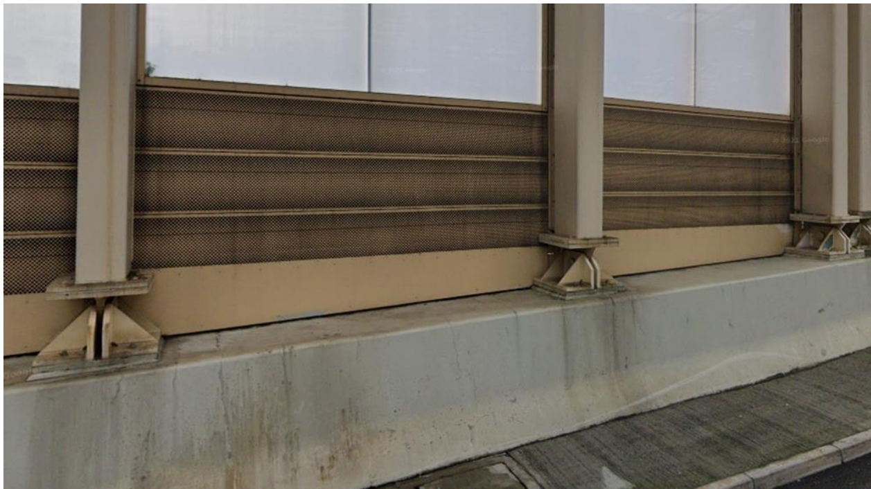
Figure 2.8.6(b) Example of Pin Support at Column Base, at Po Shun Road, Tseung Kwan O
