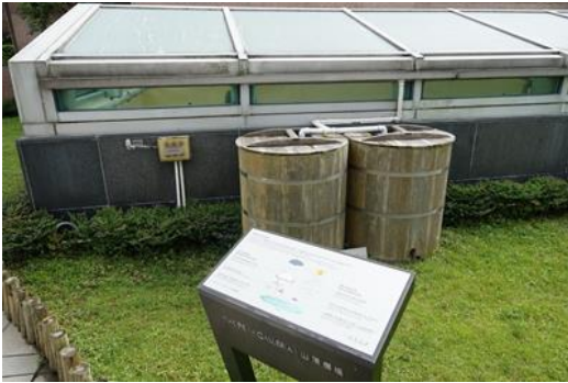
Photo 3: Rainwater harvesting system (Photo credit: Green Power)
