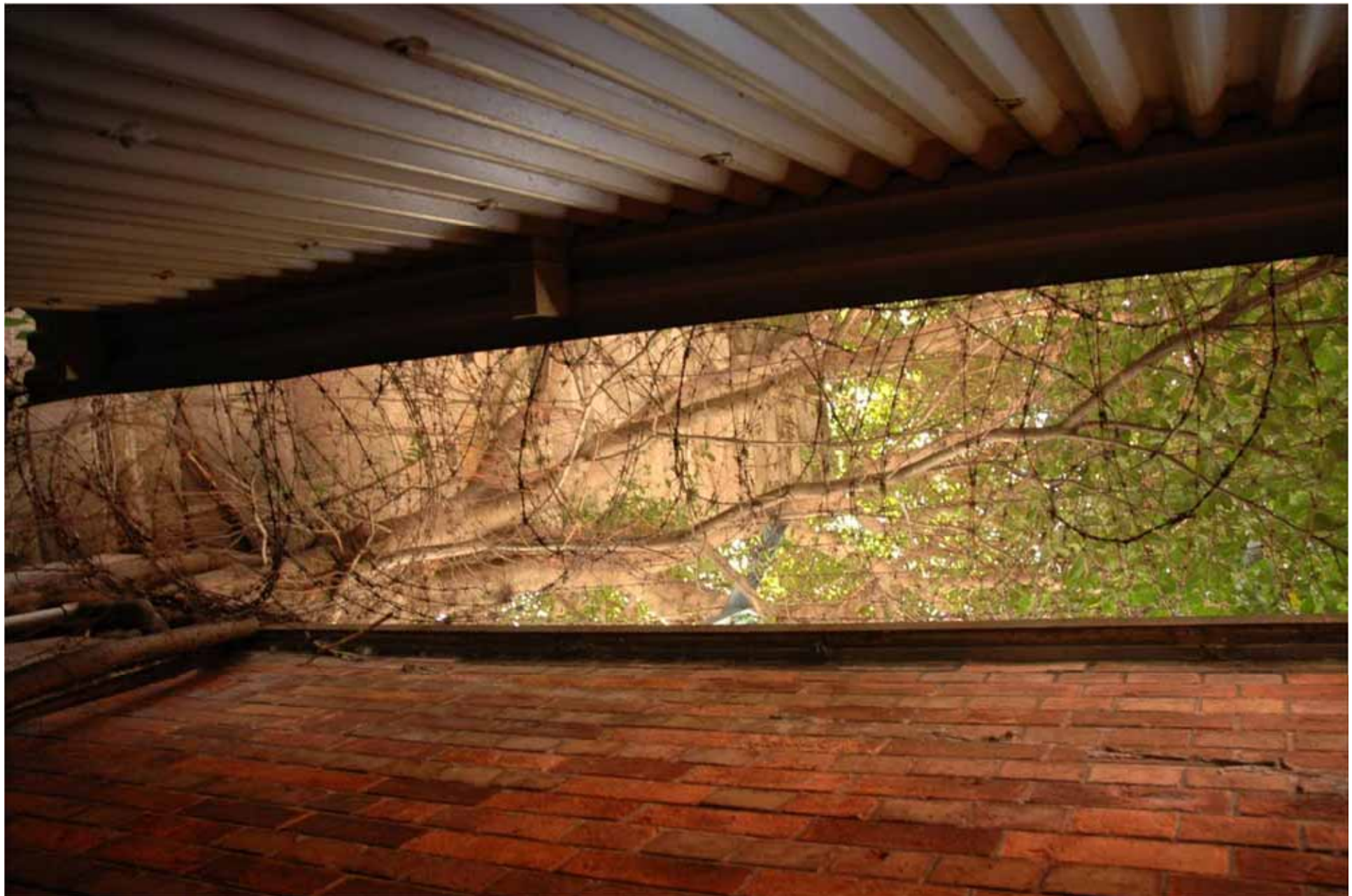
Figure 35. Looking upwards in the narrow alley where T10 is located shows its relation to the brick wall along the perimeter at Old Bailey Road and the stone retaining wall.
