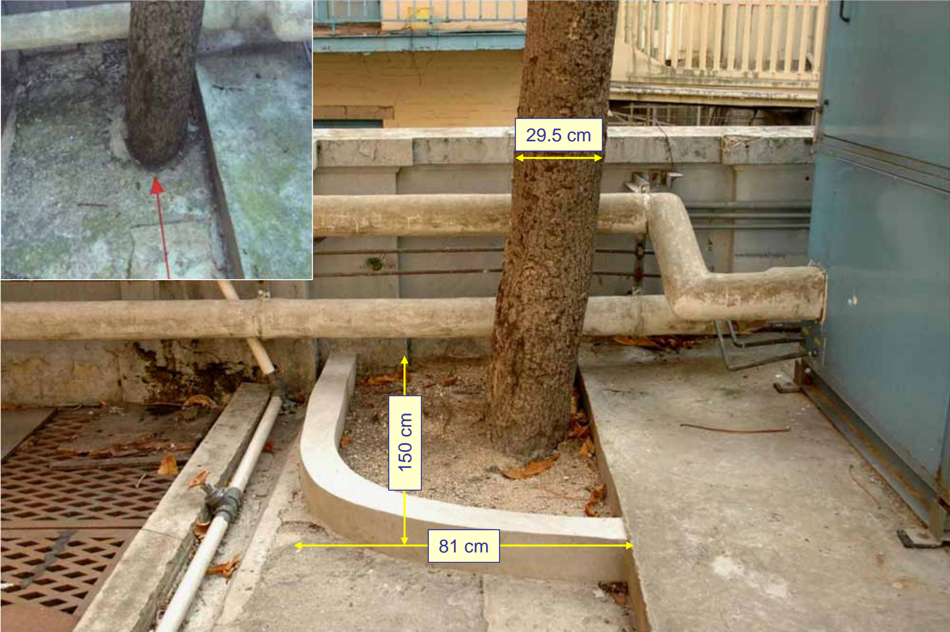
Figure 9. T1 was previously sealed by concrete to the trunk base (inset) before damage by Typhoon Fengshen. A new small tree pit has since been installed to improve soil condition.
