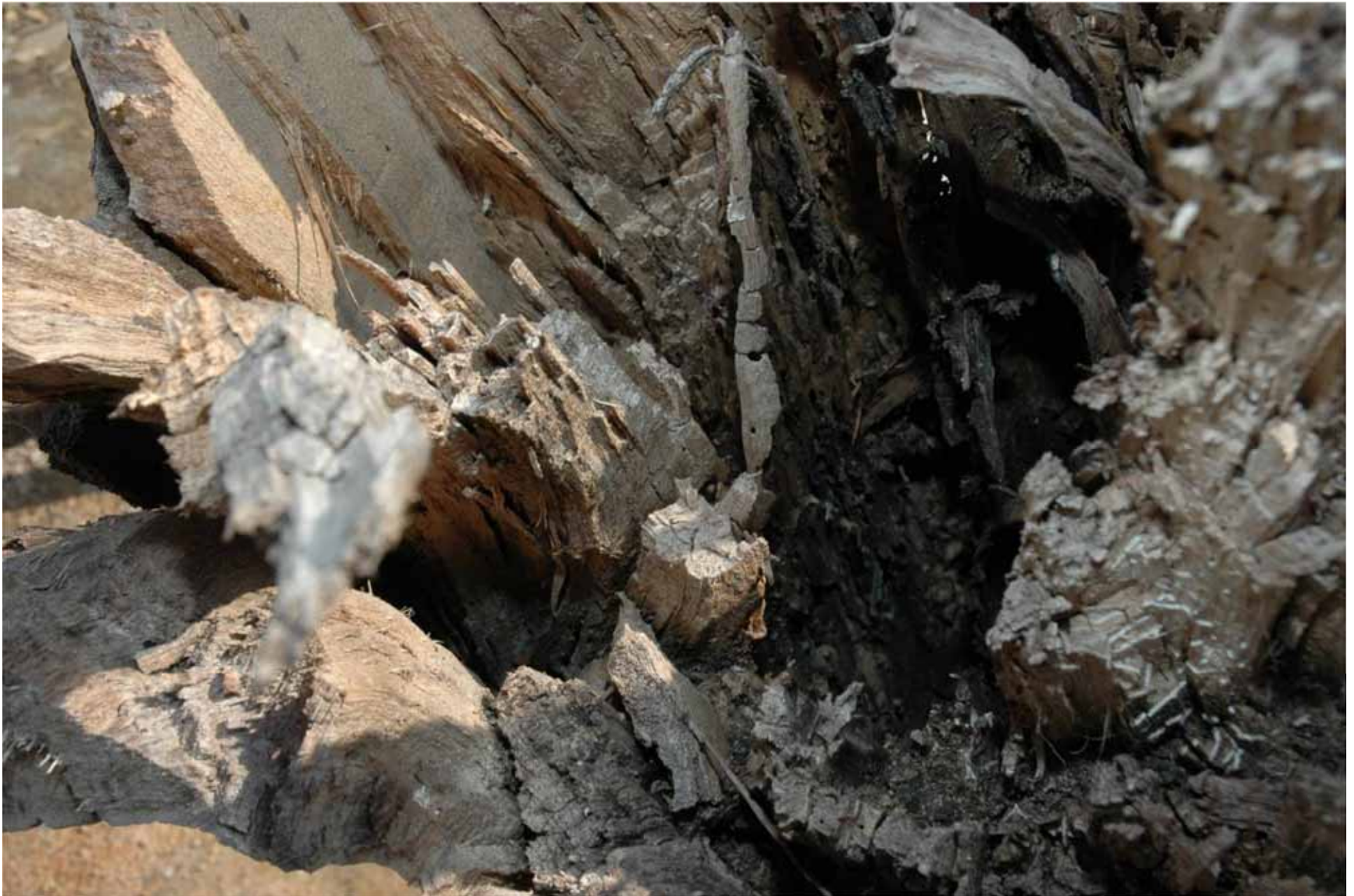
Figure 31. An interior view of the cavity in the T4 stump shows its longitudinal orientation and the degraded wood on its walls.
