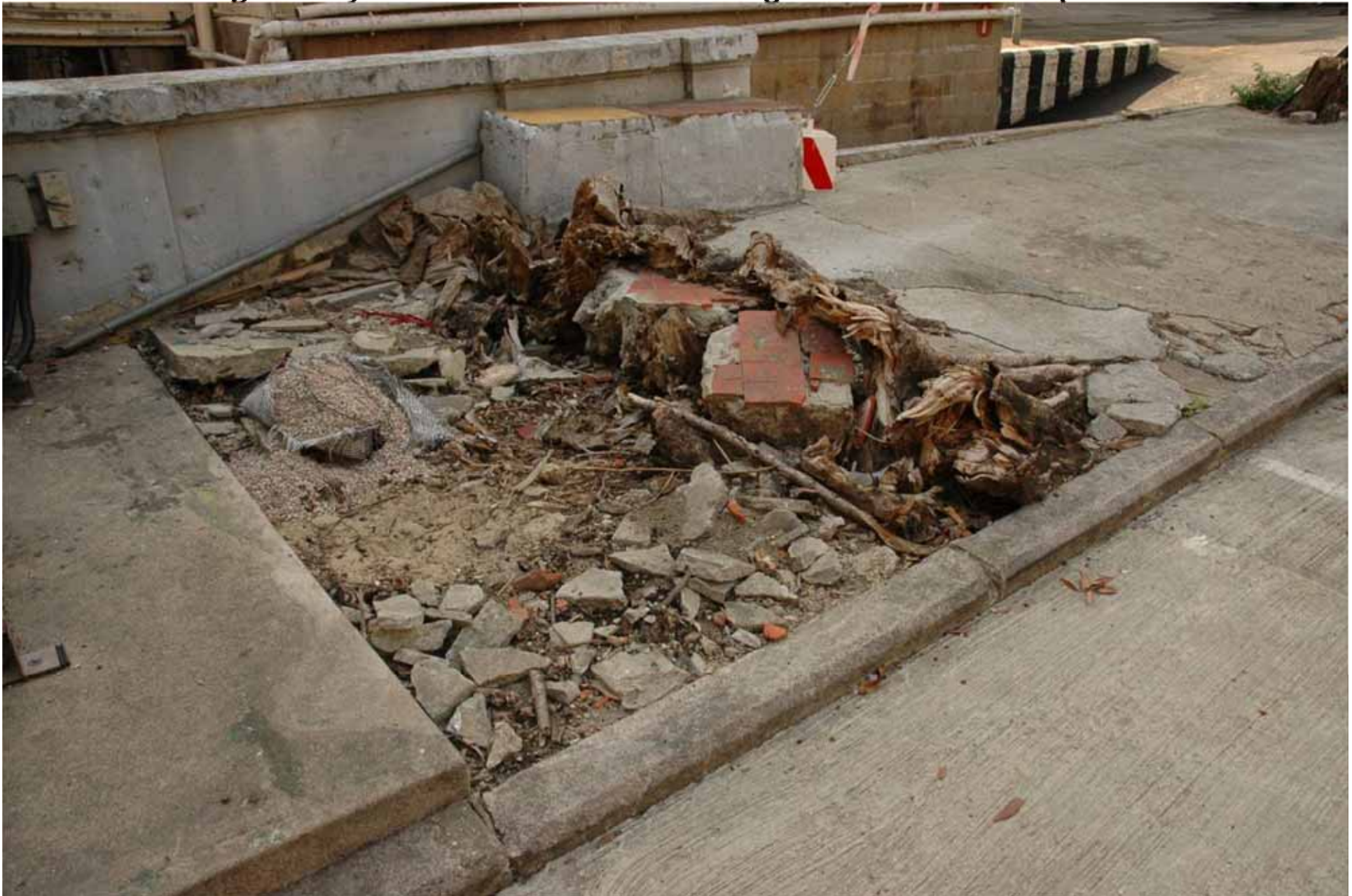
Figure 14. T2 was not provided with a proper tree pit, with concrete paved to the trunk base sealing the soil from air and water access. Old paving fragments (red tiles) engulfed by the tree in the course of its growth have been exposed.
