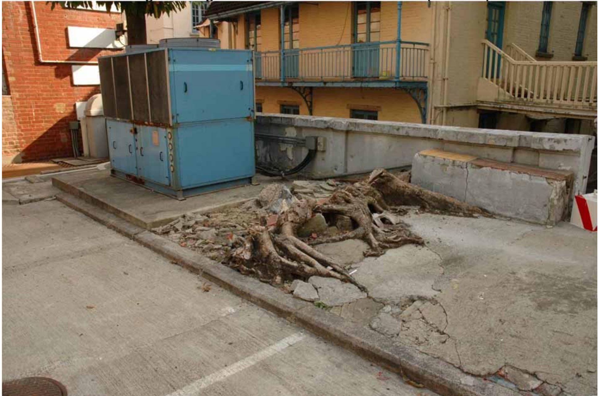
Figure 13. Remains of T2 which was snapped at the trunk base by Typhoon Fengshen. The remnant roots are found mainly on the south side; roots on the north were probably damaged during installation of the air conditioner (blue box).
