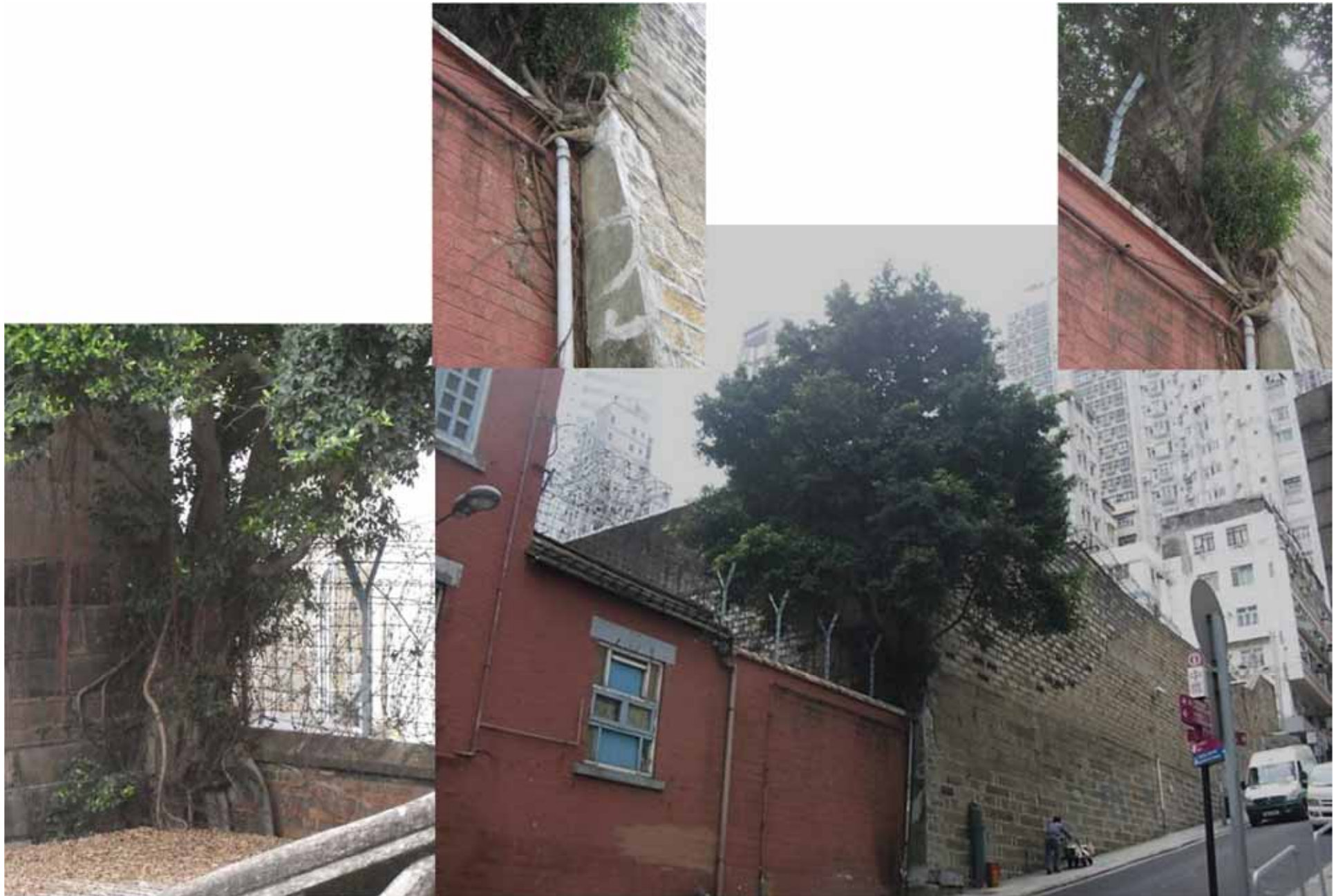
Figure 38. The condition of T10 on 17 March 2011.
