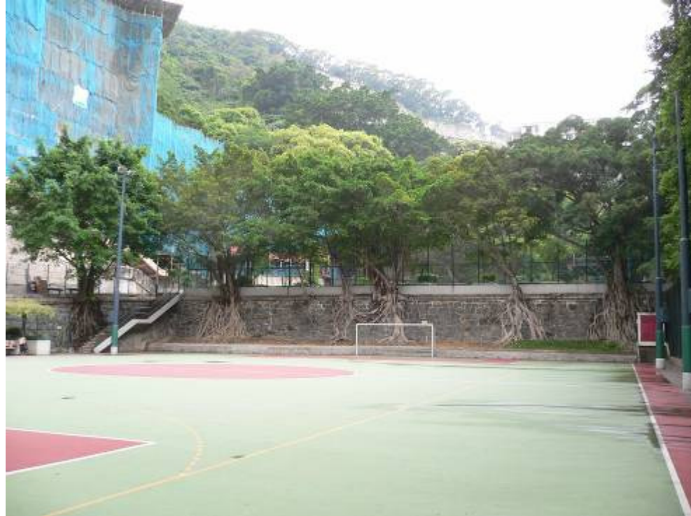
The masonry wall dividing the upper and lower portions of the playground
