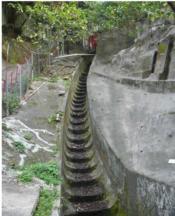
Drainage Channel (at the west of Bayanihan Kennedy Town Centre)
