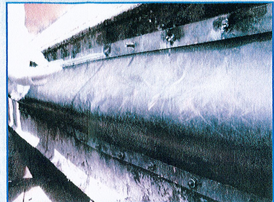
Rubber gaskets installed over the steel angles for the first field trial for Container A
