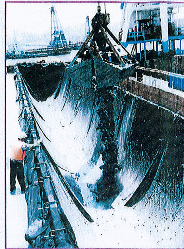
Filling of container with marine sediments by a grab hoisted by the derrick lighter
