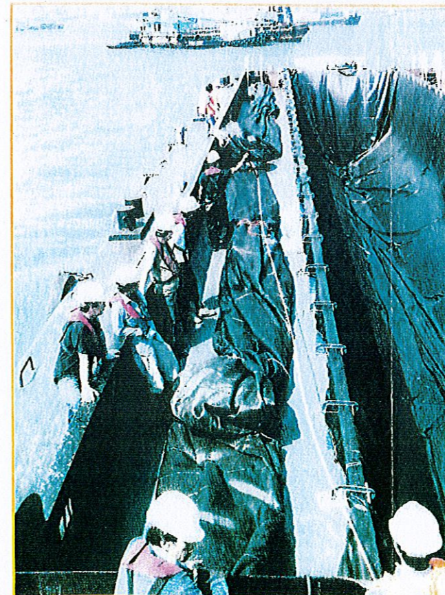
Slip sheets placed, container laid out besides the hopper and ready to be installed
