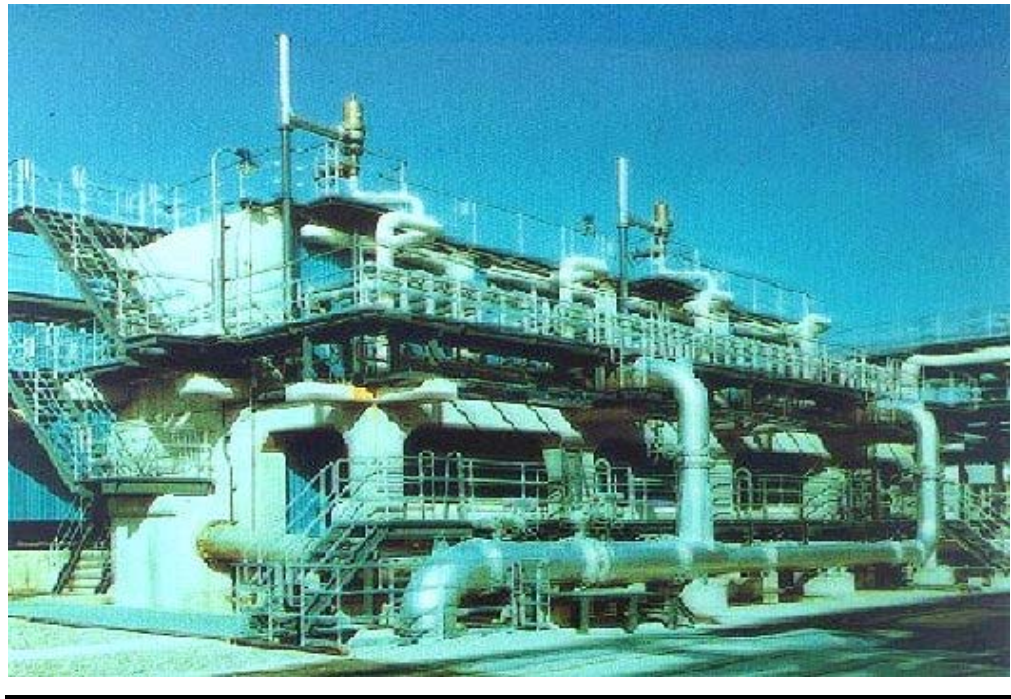
Figure 1.3 Typical Open Rack Vaporiser
