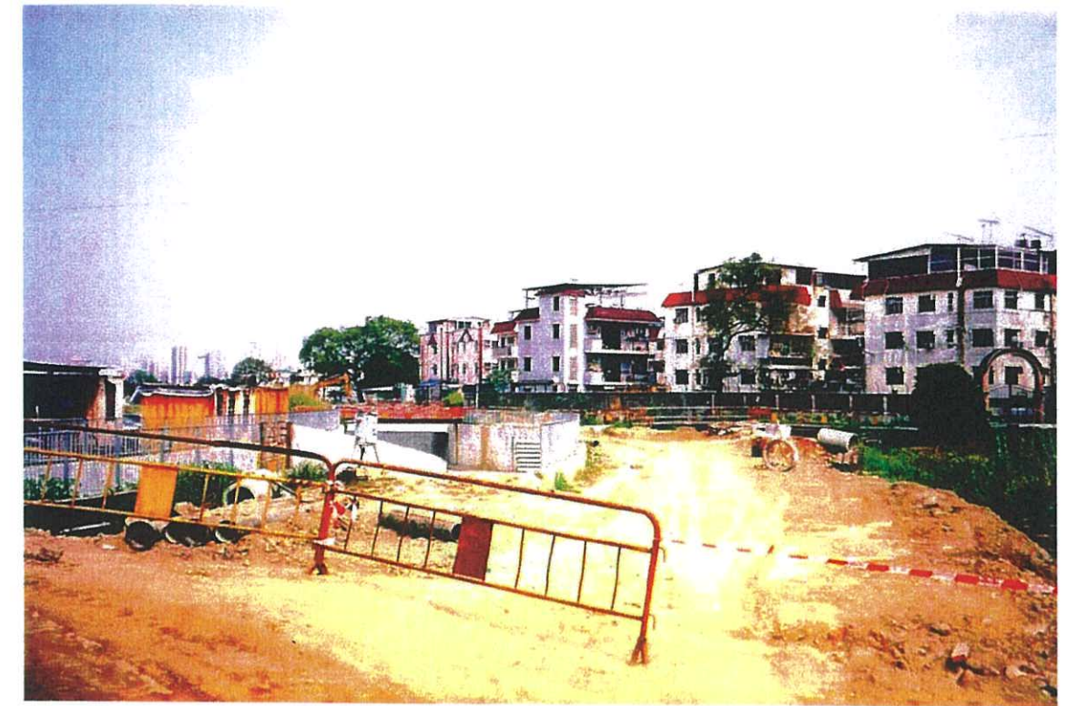
PV42: View north along Sham Chung Channel under construction with residential VSR's in background.
