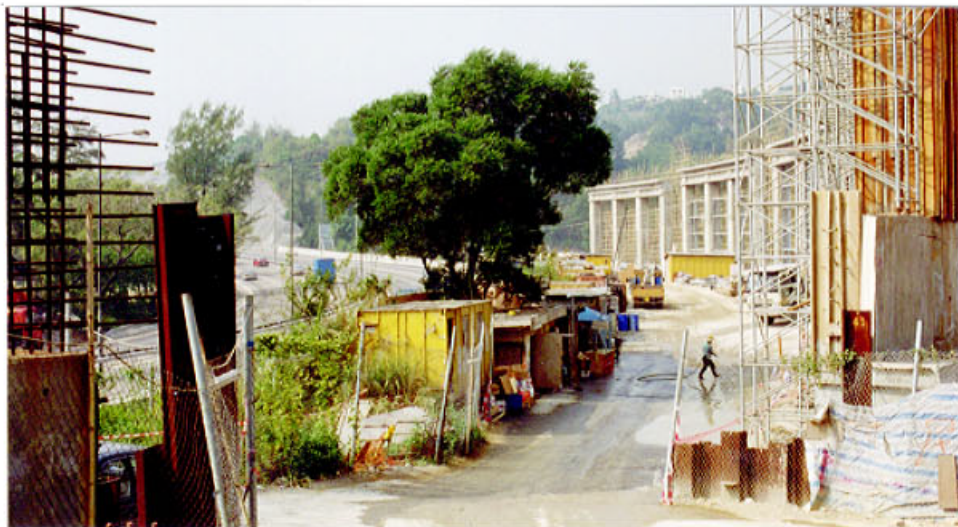
Photograph C LCU 6: SEWERS ALIGNED UNDER ROADS / FOOTPATHS ADJACENT TO NEW RESIDENTIAL DEVELOPMENT
