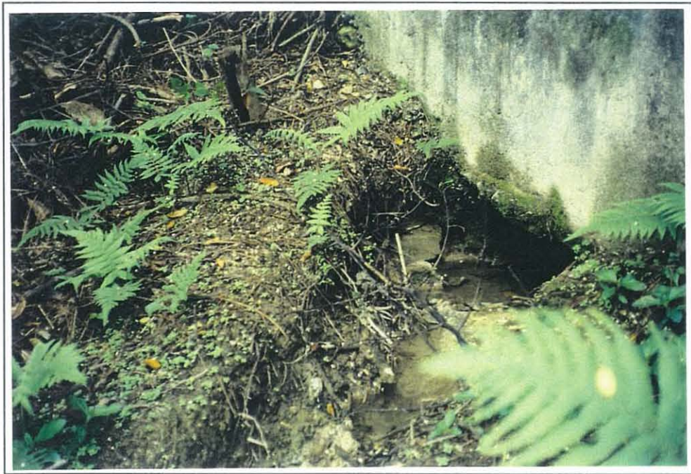
Plate 12.4 Mouth of Sludge Disposal Pipe - Tai O
