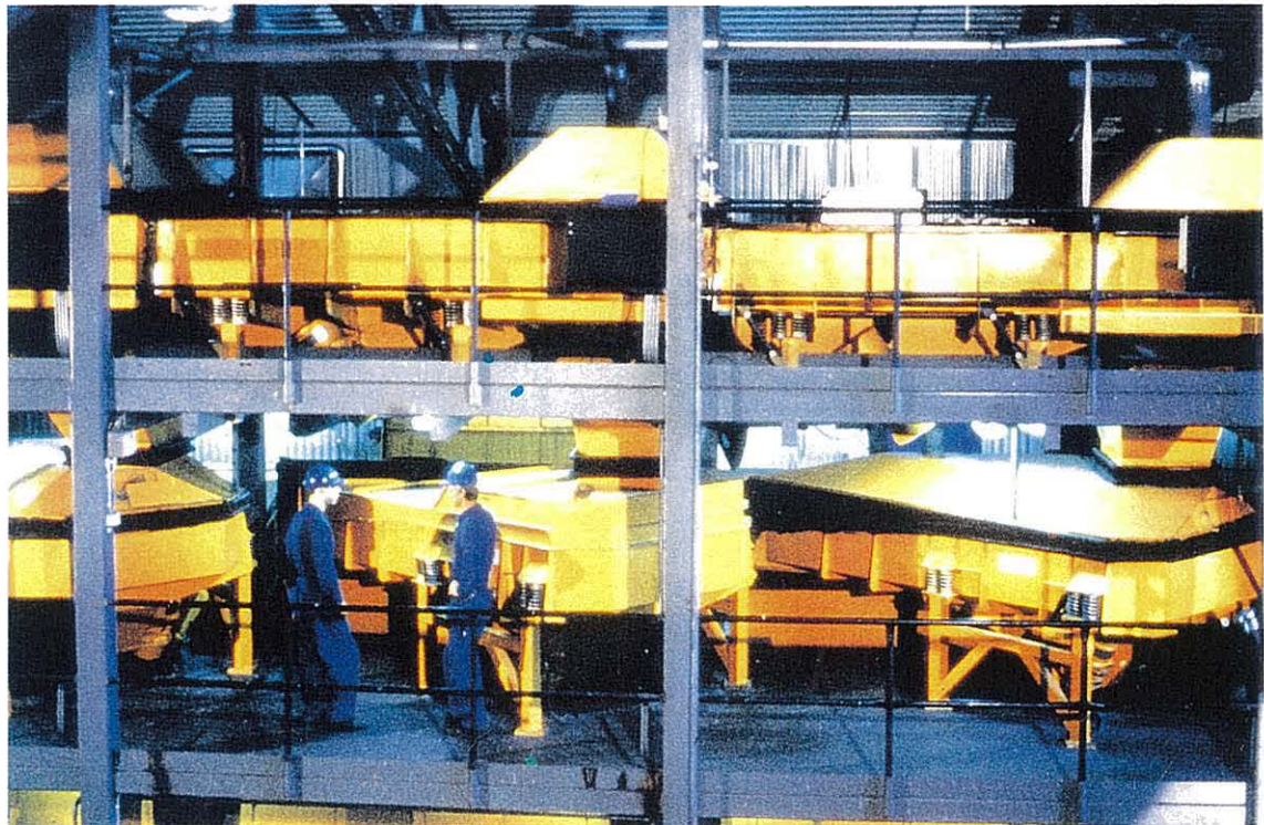
INTERNAL VIEW OF BRINI PLANT SHOWING SHREDDED WASTE CLASSIFIERS
