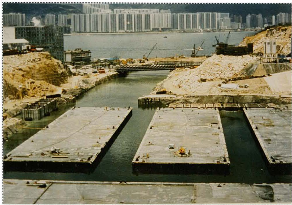
Plate No 2.2 - Construction of the road/rail Eastern Harbour Crossing immersed tube units; Cha Kwu Ling, East Kowloon 1988. The photograph shows the flooded basin prior to the completed units being floated out.
