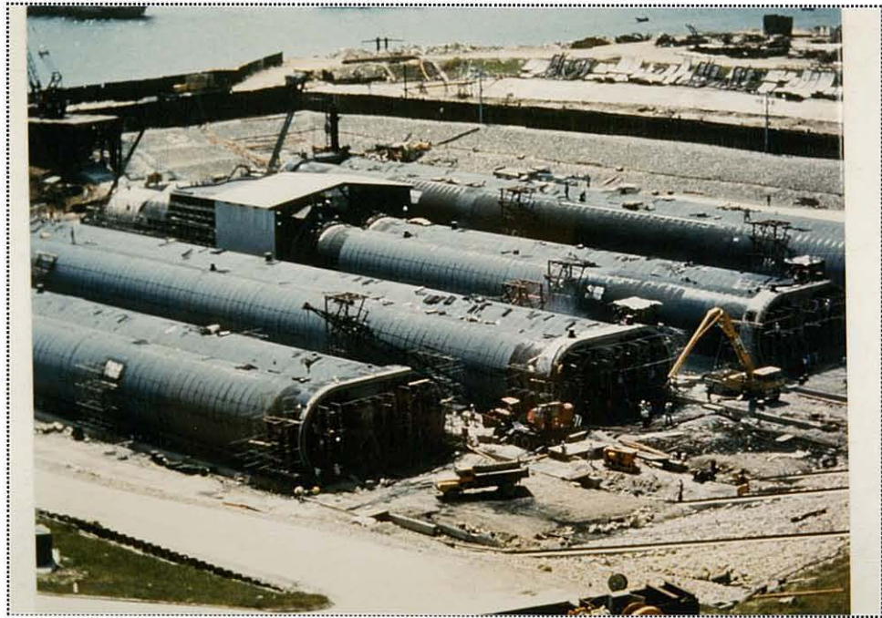
Plate No 2.1 - Construction of the MTR Tsim Sha Tsui to Admiralty immersed tube units; Northpoint, Hong Kong Island 1977-1978. The size of the units and casting basin are similar to that proposed for Pok Tung Wan Quarry site.
