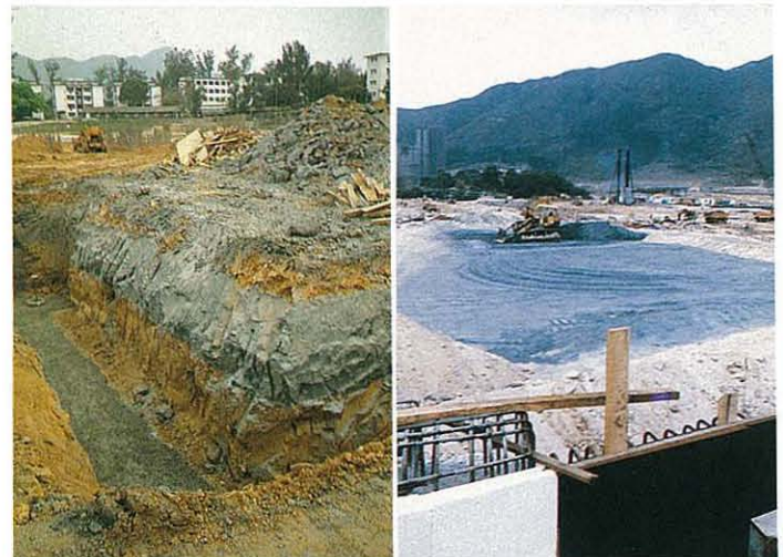
Foundation excavation through PFA fill for Tuen Mun housing blocks. PFA fill for road embankments in Tuen Mun. 屯門屋邨地基煤灰填地開掘工程 屯門煤灰填築路堤
