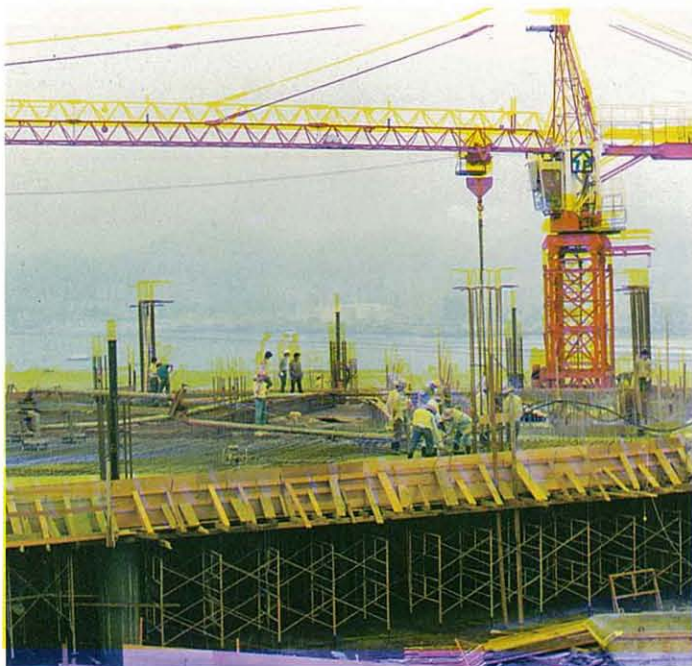
Formwork preparation for one of the lower floors. 其中一較低底盤的模板準備。
