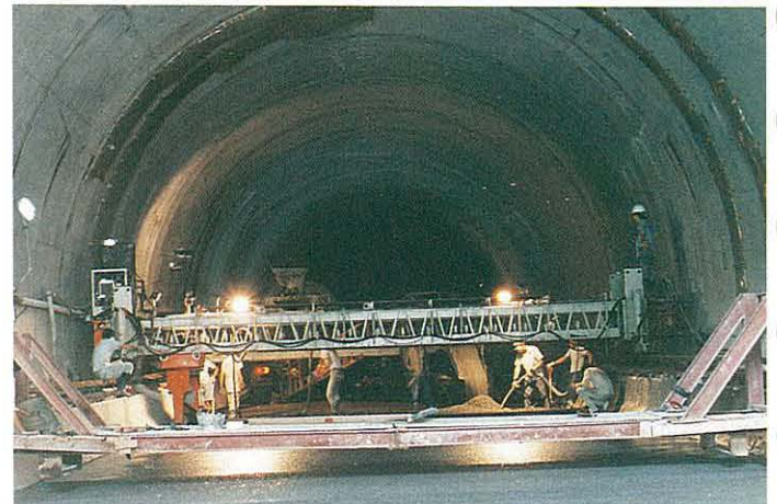
PFA concrete in the Route 5 tunnel linings and roads. 煤灰混凝土用於5號公路隧道襯壁及道路
