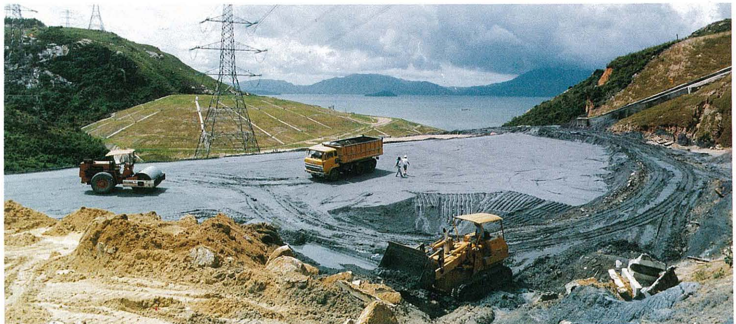
Typical operations at a PFA fill site. 煤灰填築地盤施工情景
