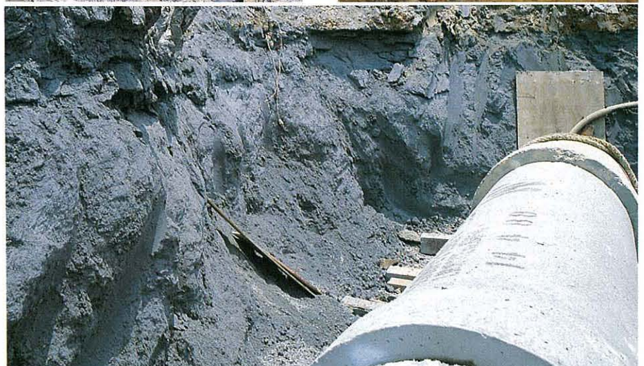
Piling, trenching and handling the PFA fill presented no difficulties at Tuen Mun. 煤灰填料不會在打樁、開溝及處理上引起不便
