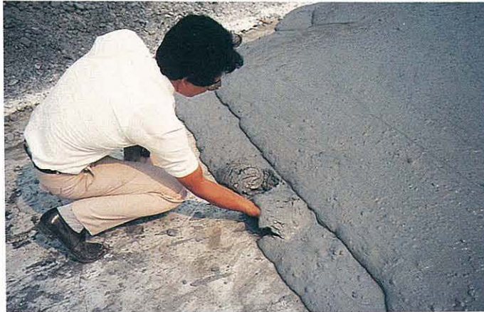
Flowable PFA fill, using 5% cement and seawater, had a strength of 1 MPa at 1 day.
