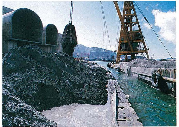
Marine reclamation for the Eastern Harbour Crossing using PFA as a lightweight fill. 東區海底隧道填海區使用煤灰作為輕質填料
