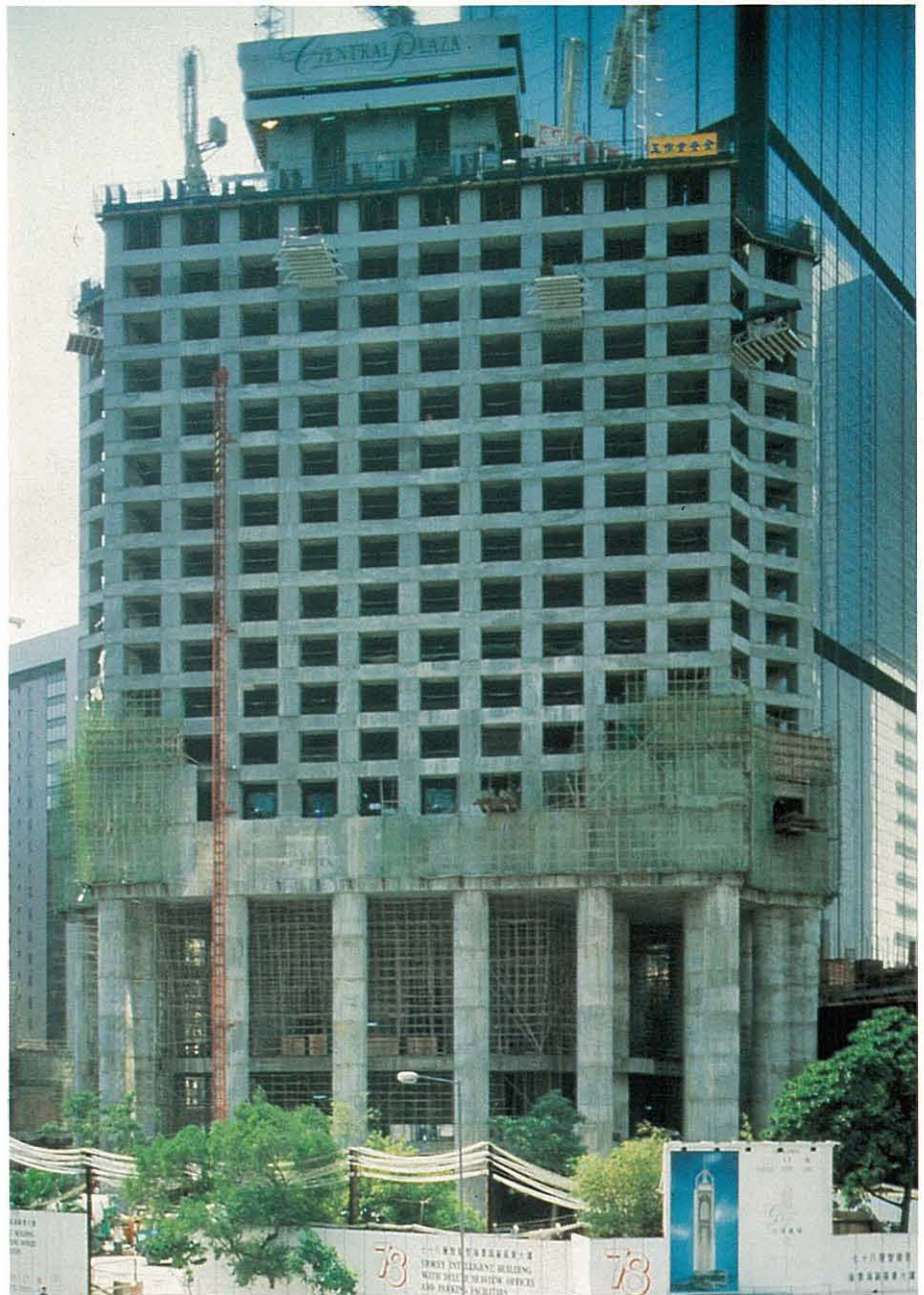
A fast construction rate was achieved using reinforced concrete. 利用鋼筋混凝土使工程進度加快。
