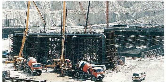
PFA concrete for the Eastern Harbour Crossing immersed tube units. 煤灰混凝土用於東區海底隧道的海底管道
