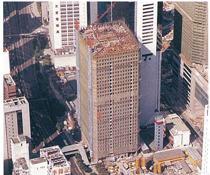
Construction of the Harbour Road Government Offices using PFA concrete. 煤灰混凝土用於建築港灣道政府合署
