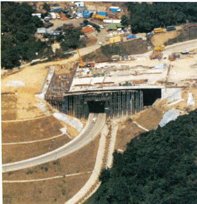
Approach structures used large volumes of PFA concrete. 採用大量煤灰混凝土的引道結構
