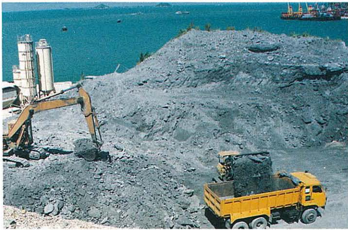
Excavation of PFA fill 5 years after placing. 煤灰填地澆築五年之後開挖情景
