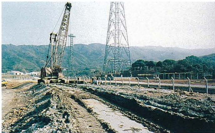
The slurry cut-off wall at Tsang Tsui used a PFA/cement/bentonite mix. 煤灰／水泥／斑脫土漿曾阻隔火警
