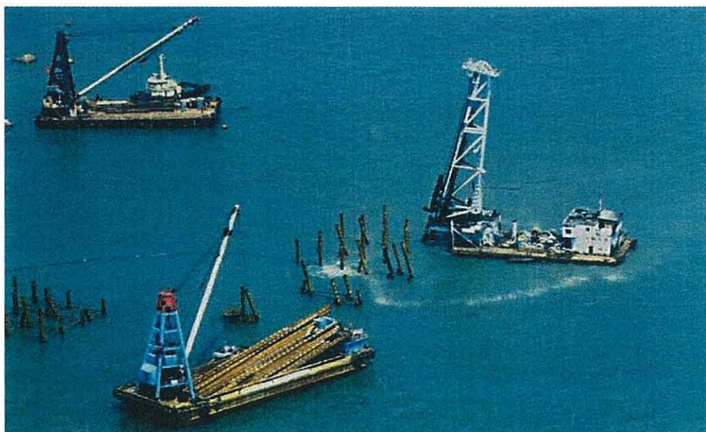
An air bubble curtain was developed to reduce underwater noise from percussive piling.
