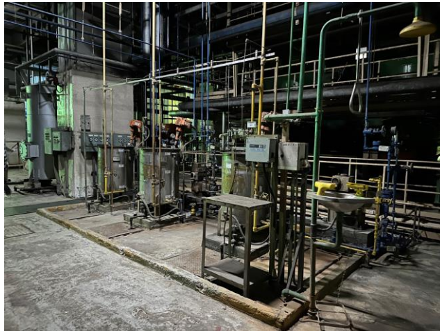
Photo 22: Chemical dosing system at L3
