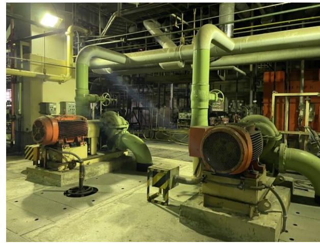
Photo 44: Bearing cooling water pump
