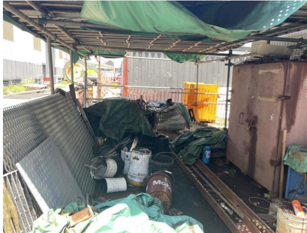
Photo 80: A storage area of equipment with oil stains and emptied chemical containers in place
