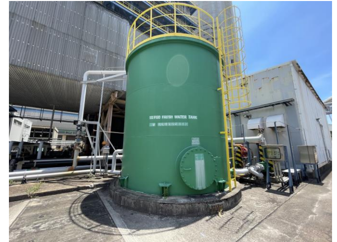
Photo 69: Water tank for the FGD plant
