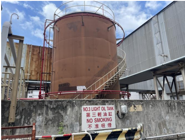
Photo 73: Unit 3 Light Oil Tank
