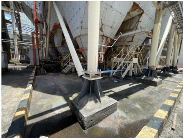
Photo 64: Ash hopper of the electrostatic precipitator system
