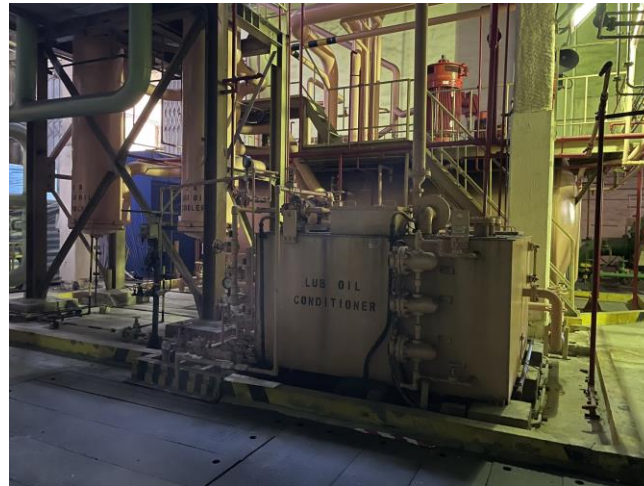
Photo 29: Lubrication oil conditioner and coolers at L2
