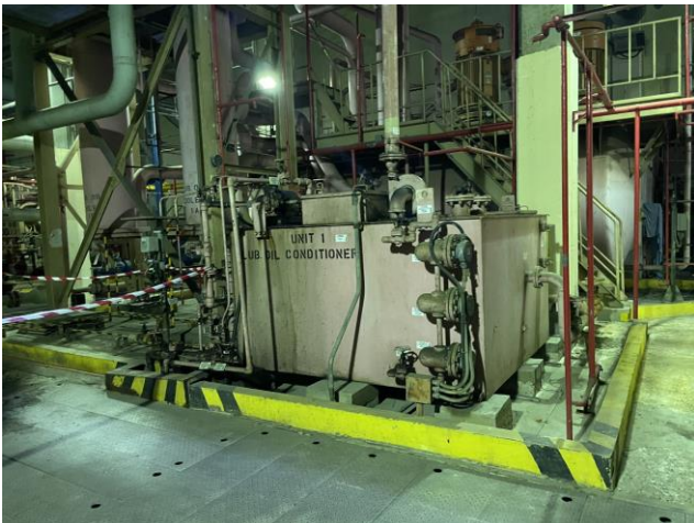
Photo 28: Lubrication oil conditioner and coolers at L1
