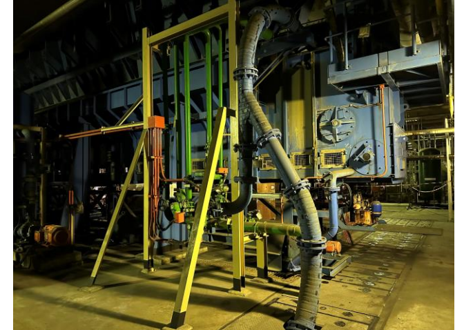
Photo 6: Boiler area and submerged scraper conveyor
