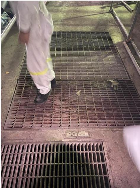
Photo 10: A blown down drain pit
