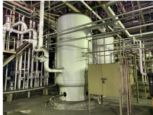
Photo 41: Boiler air receiver units
