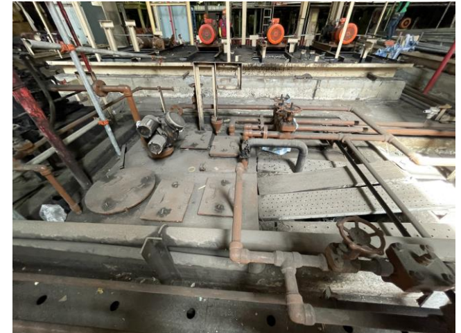
Photo 12: A fuel oil drain tank
