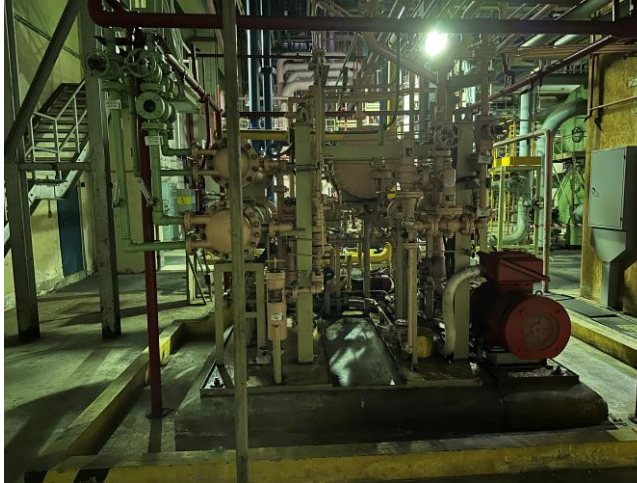
Photo 35: Seal oil supply unit at L3
