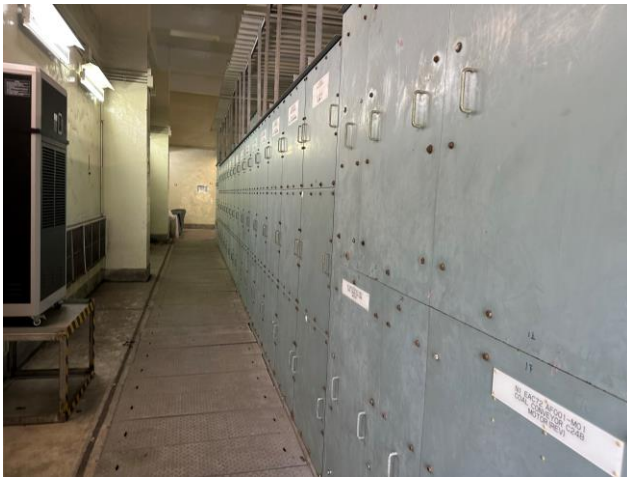
Photo 88: Switchgear room in the GT57 & Coal Jetty Electrical Equipment Building
