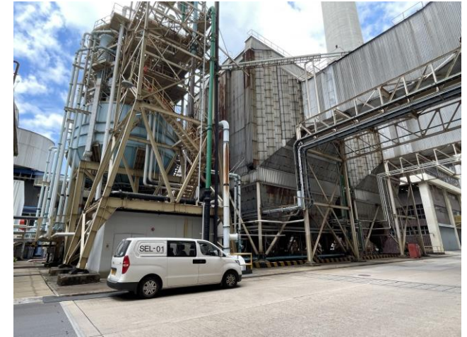
Photo 63: Electrostatic precipitator systems connecting from the Main Station Building for L1 to L3
