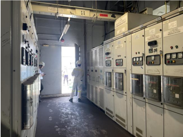
Photo 79: Switchgear room in Unit 2 FGD Electrical and Control Equipment Building
