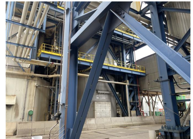
Photo 66: The absorber of the Flue Gas Desulphurisation (FGD) plant
