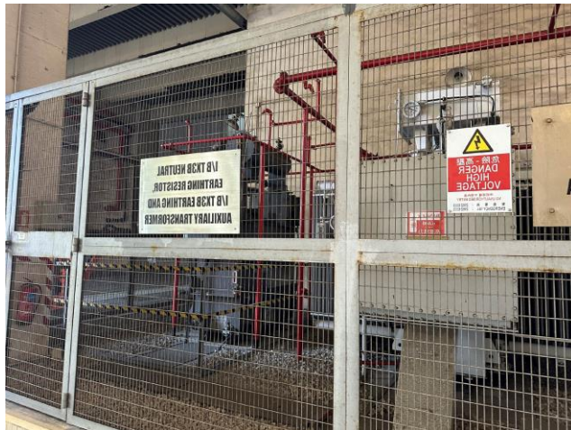
Photo 58: Transformer along the Main Station Building
