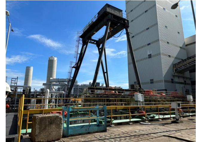
Photo 84: Overview of the circulating water system and Junction Tower T16 at the back
