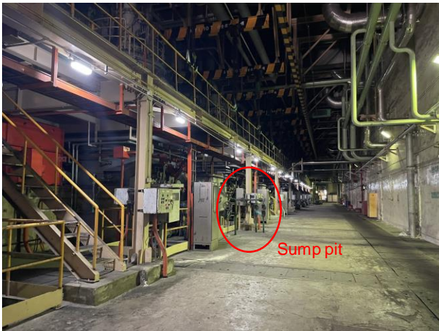
Photo 16: A series of coal grinding mills along the Main Station Building and sump pit
