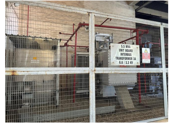
Photo 57: Transformer along the Main Station Building
