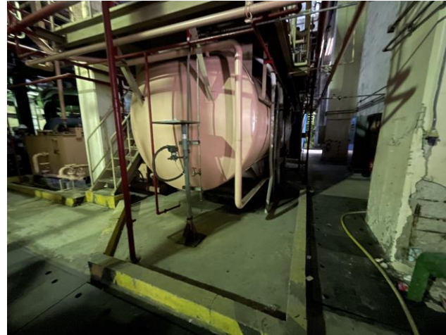
Photo 26: Main oil tank at L2
