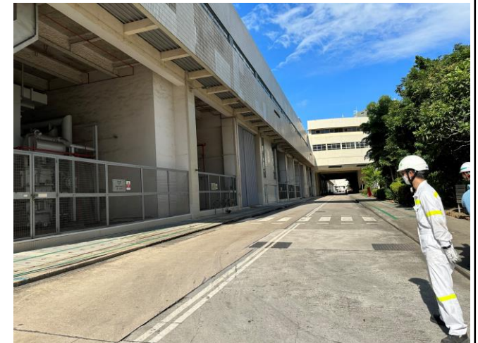
Photo 60: Transformer units along the Main Station Building
