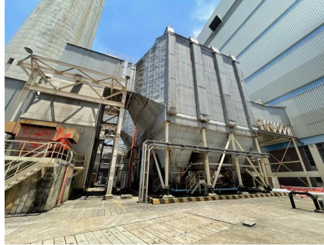
Photo 62: Electrostatic precipitator systems connecting from the Main Station Building for L1 to L3
