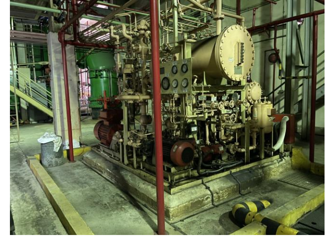
Photo 33: Seal oil supply unit at L2
