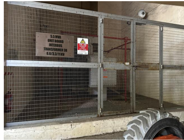
Photo 59: Transformer along the Main Station Building
