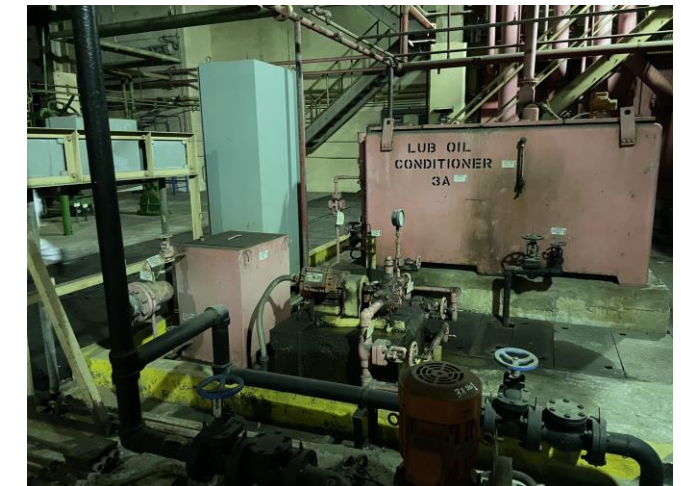
Photo 30: Lubrication oil conditioner, oil pumps and sump pit at L3 with oil stains observed
