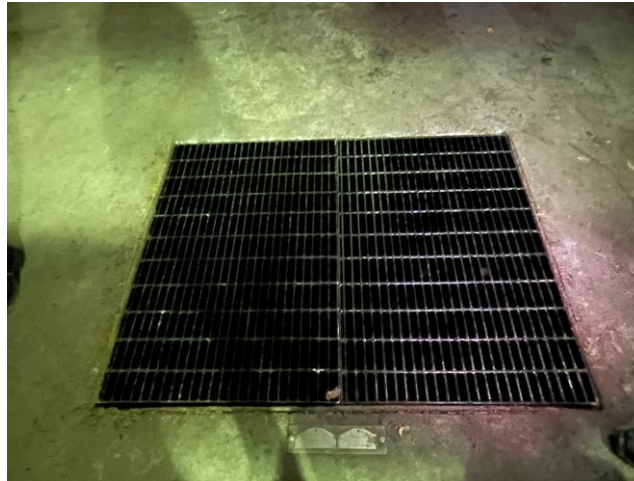
Photo 11: A blown down drain pit
