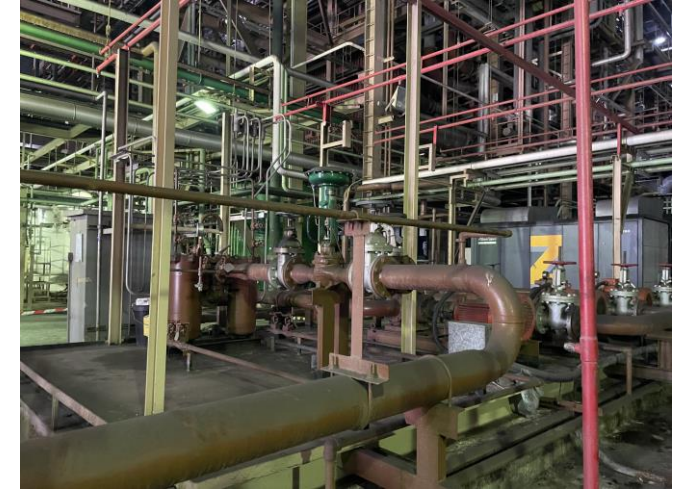
Photo 15: Fuel oil heaters
