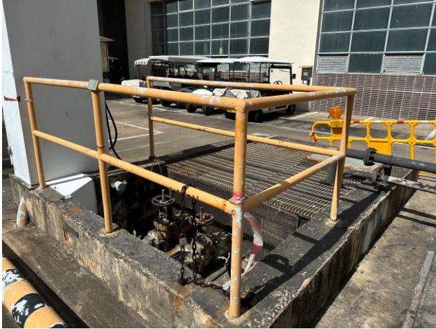
Photo 61: The oily drain sump outside the Main Station Building for L1 to L3
