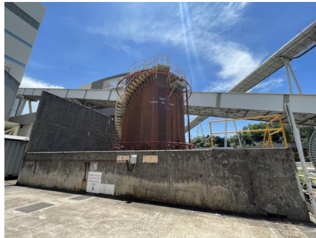
Photo 71: Secondary containment of Unit 1 Light Oil Tank
