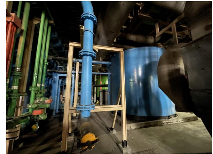
Photo 42: Water tank and overflow water tank
