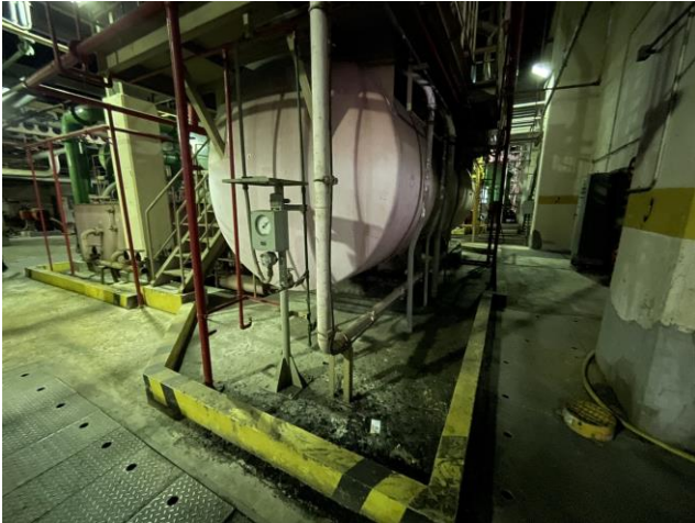
Photo 25: Main oil tank at L1
