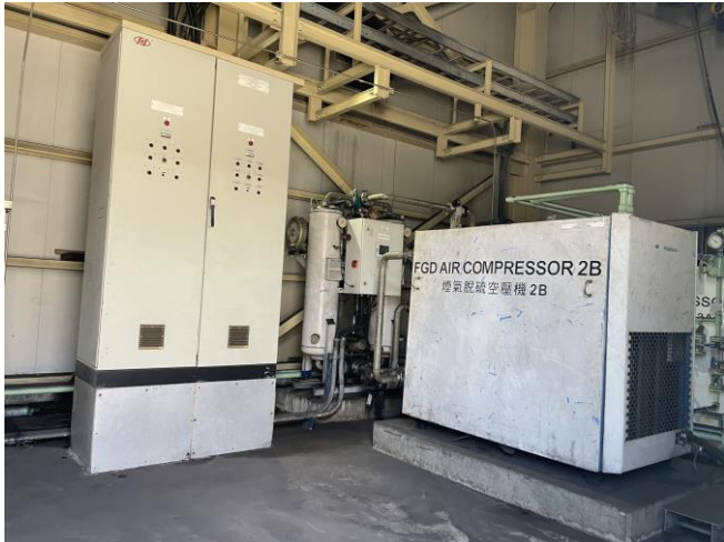
Photo 67: The air compressor units of the Flue Gas De-sulphurisation (FGD) plant
