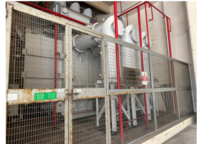
Photo 54: Transformer along the Main Station Building
