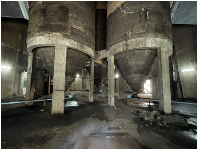
Photo 70: Inside view of the chimney with mixture of dirt and stagnant water observed
