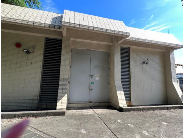
Photo 85: Cooling water system control room
