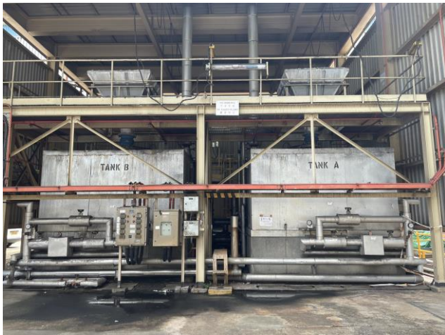
Photo 82: Two Sulphur melting / store tanks underneath a shelter with oil stain observed.
