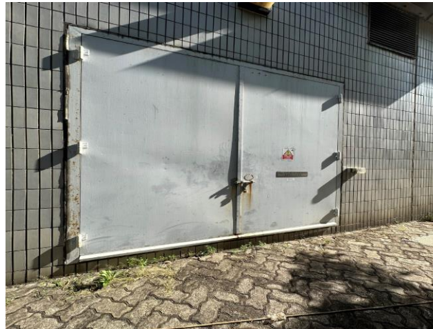
Photo 89: Transformer room in the GT57 & Coal Jetty Electrical Equipment Building
