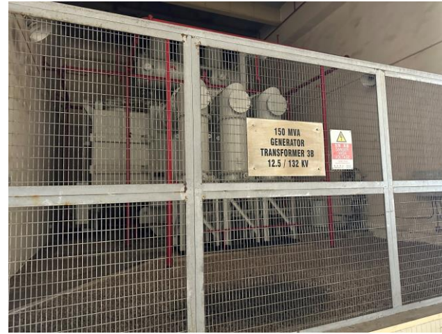
Photo 56: Transformer along the Main Station Building
