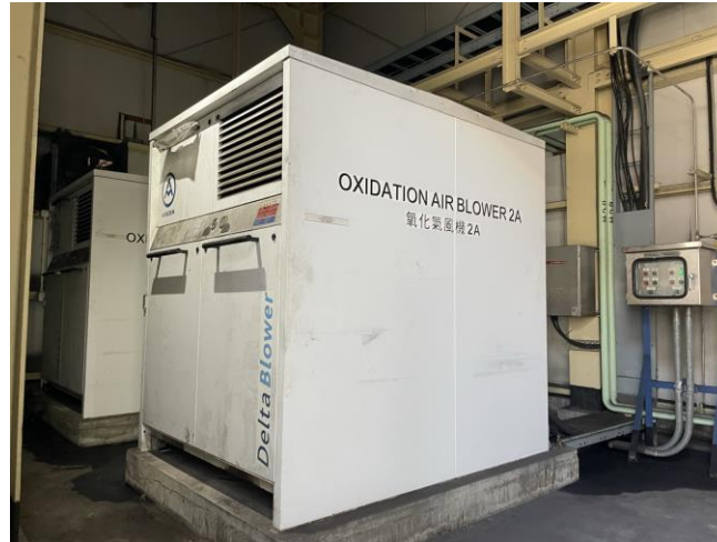
Photo 68: The oxidation air blower units of the FGD plant with oil stains observed
