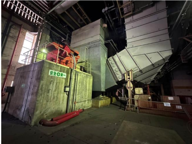
Photo 37: A forced draft fan unit
