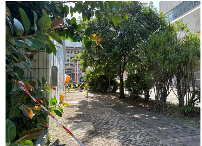
Photo 96: Brick pavers area outside the GT57 & Coal Jetty Electrical Equipment Building
