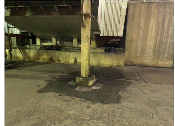
Photo 39: A oil stain near a forced draft fan unit in L2
