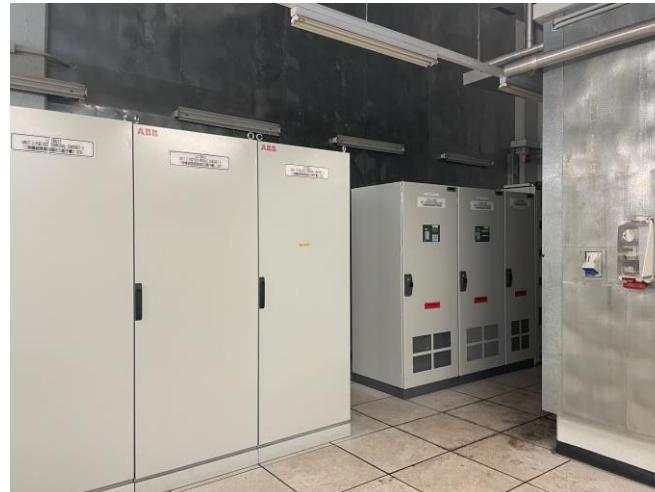
Photo 77: Control equipment room in Unit 2 FGD Electrical and Control Equipment Building
