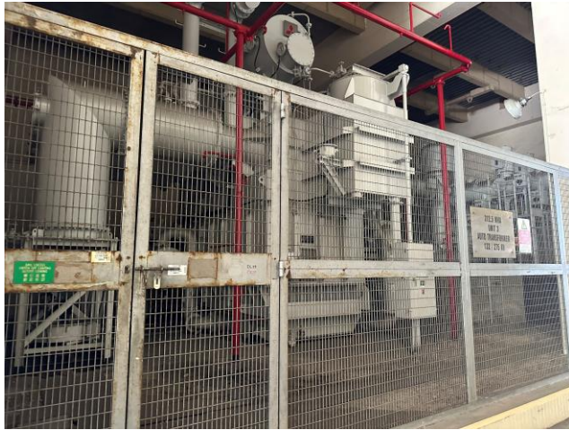
Photo 55: Transformer along the Main Station Building
