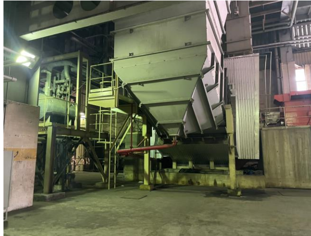
Photo 38: A oil stain near a forced draft fan unit in L2
