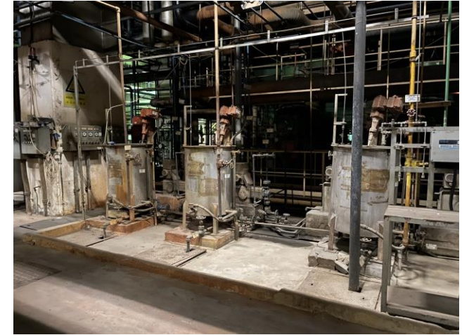
Photo 21: Chemical dosing system at L3
