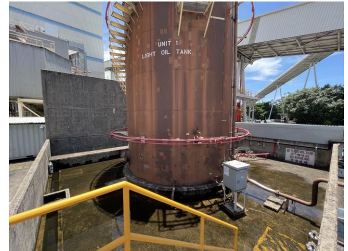
Photo 72: Unit 1 Light Oil Tank
