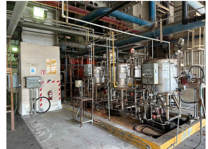
Photo 18: Chemical dosing system at L1
