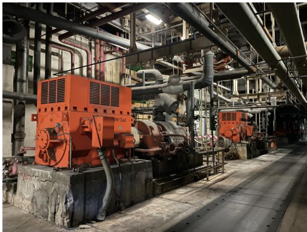
Photo 46: Boiler feed pumps
