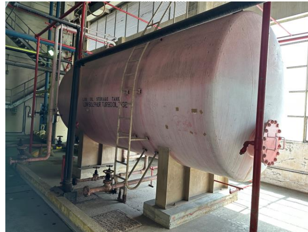
Photo 23: Lubrication oil storage tank
