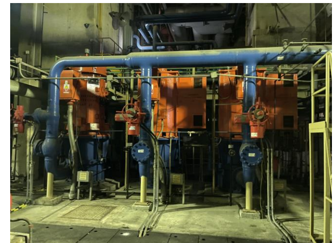
Photo 45: Condensate extraction pumps
