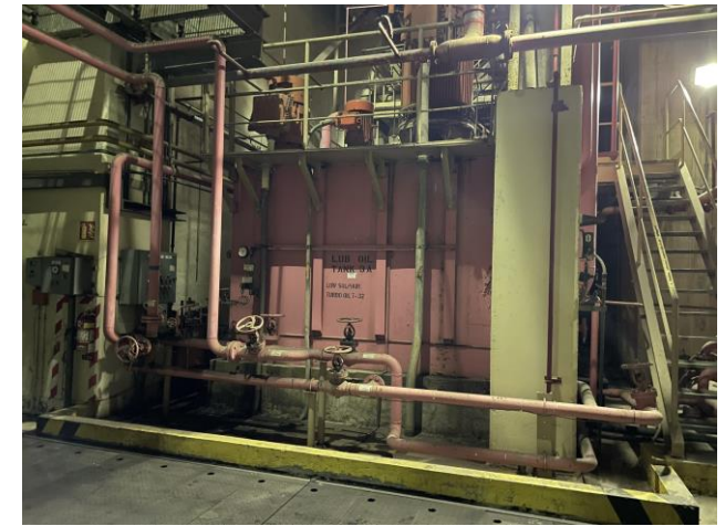
Photo 27: Lubrication oil tank at L3
