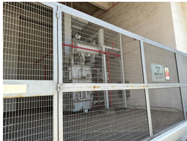
Photo 47: Transformer along the Main Station Building
