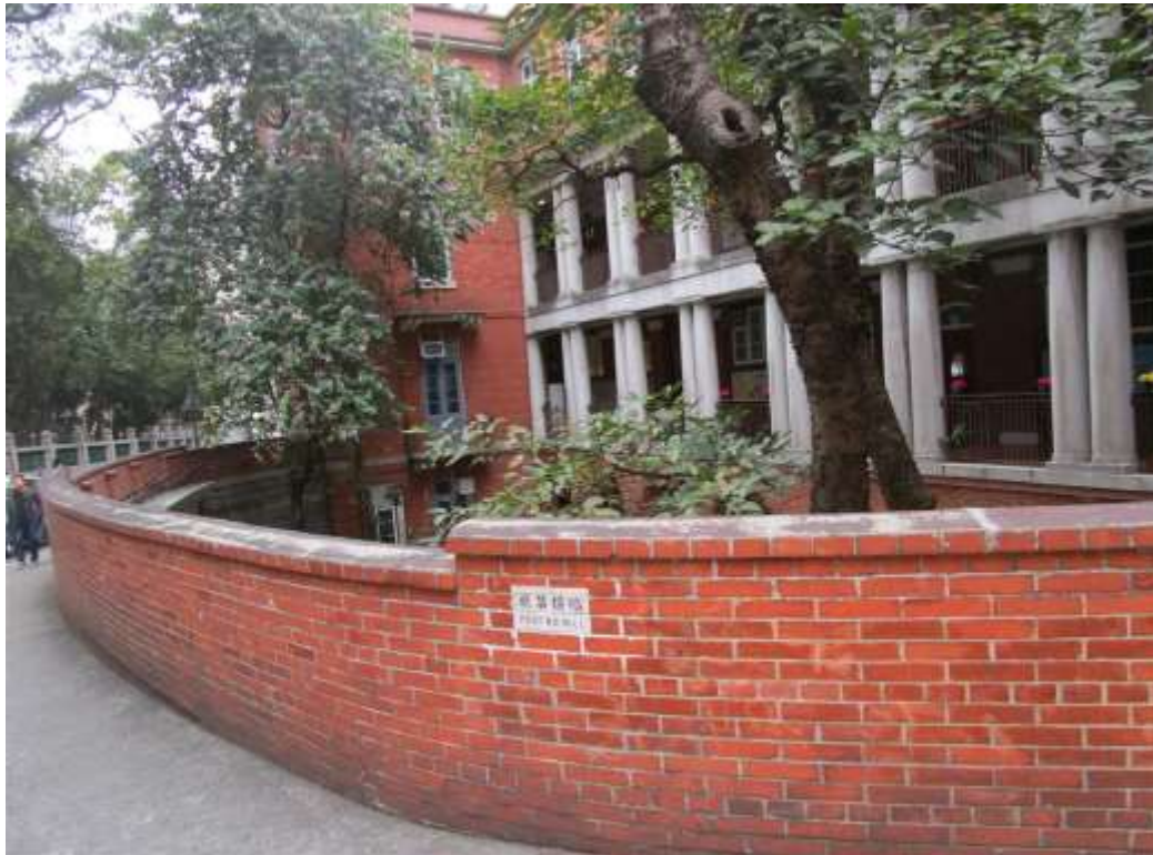
General View No. GV49 Description General view of parapet wall, south elevation
