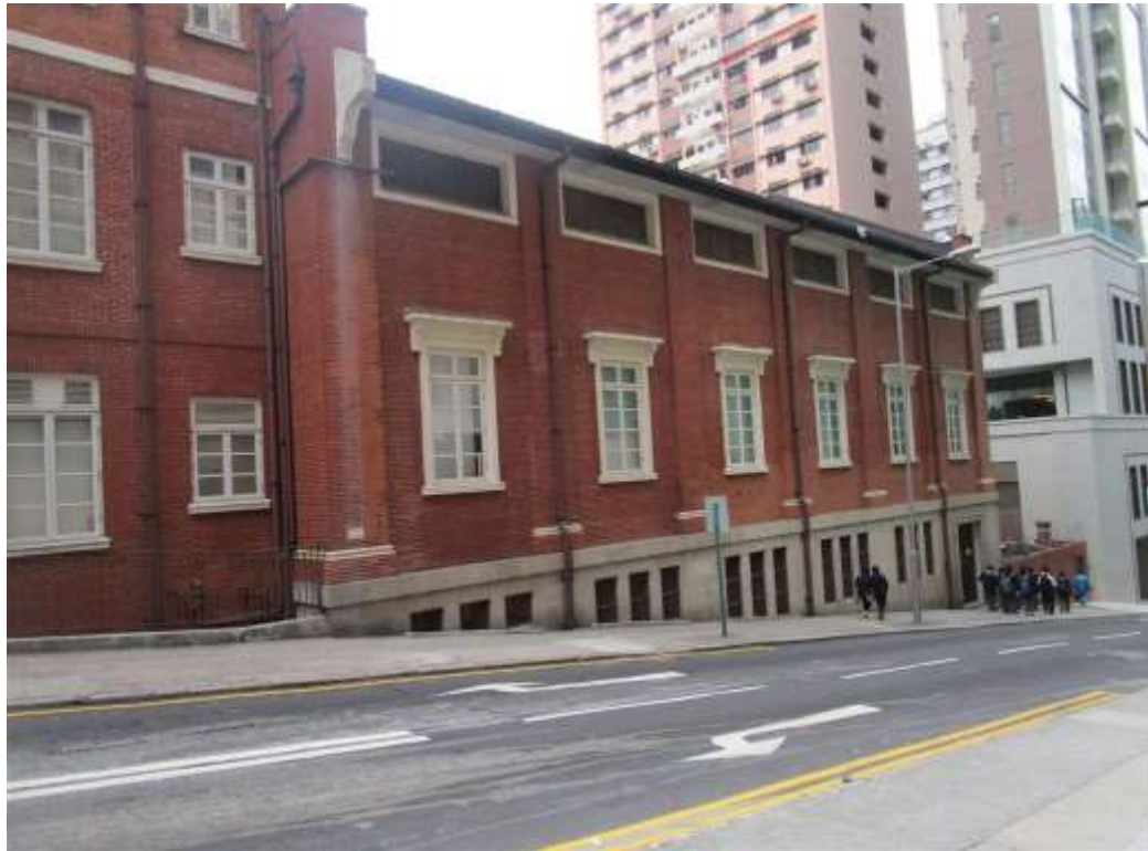
General View No. GV5 Description General view of east wing, east elevation
