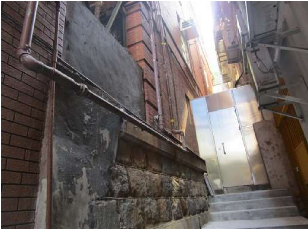
General View No. GV37 Description General view of south wing, west elevation back lane
