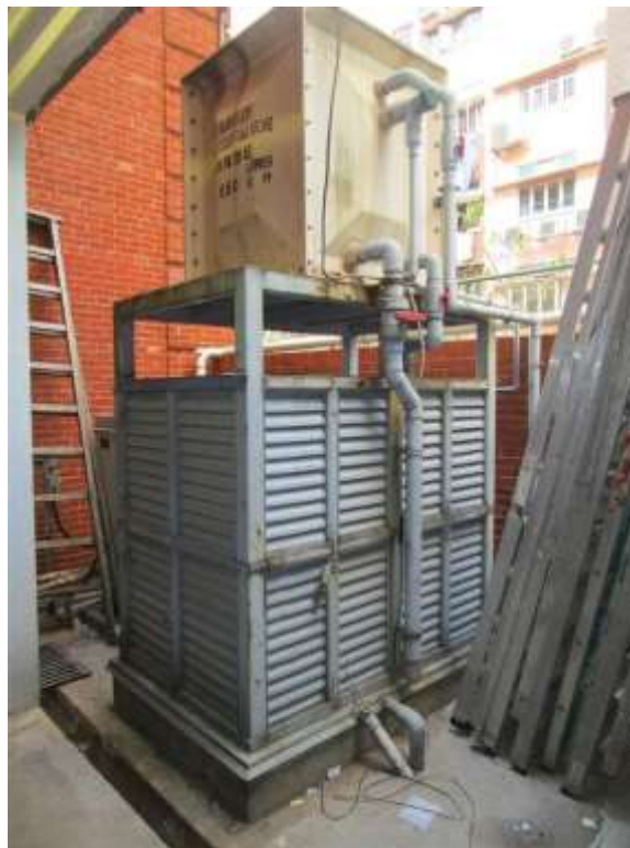
General View No. GV16 Description General view of water tank on top of north retaining wall inside staff quarter area
