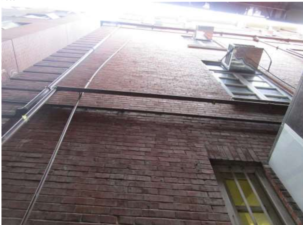
General View No. GV52 Description General view of brickwall of south wing, west elevation
