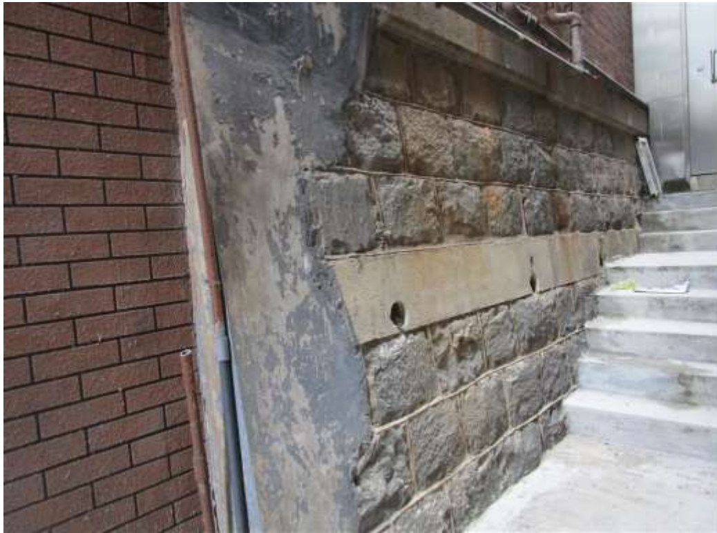
General View No. GV51 Description General view of retaining wall, west elevation
