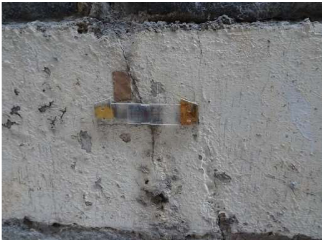
General View No. GV14 Description General view of tell-tale crack gauge on north retaining wall
