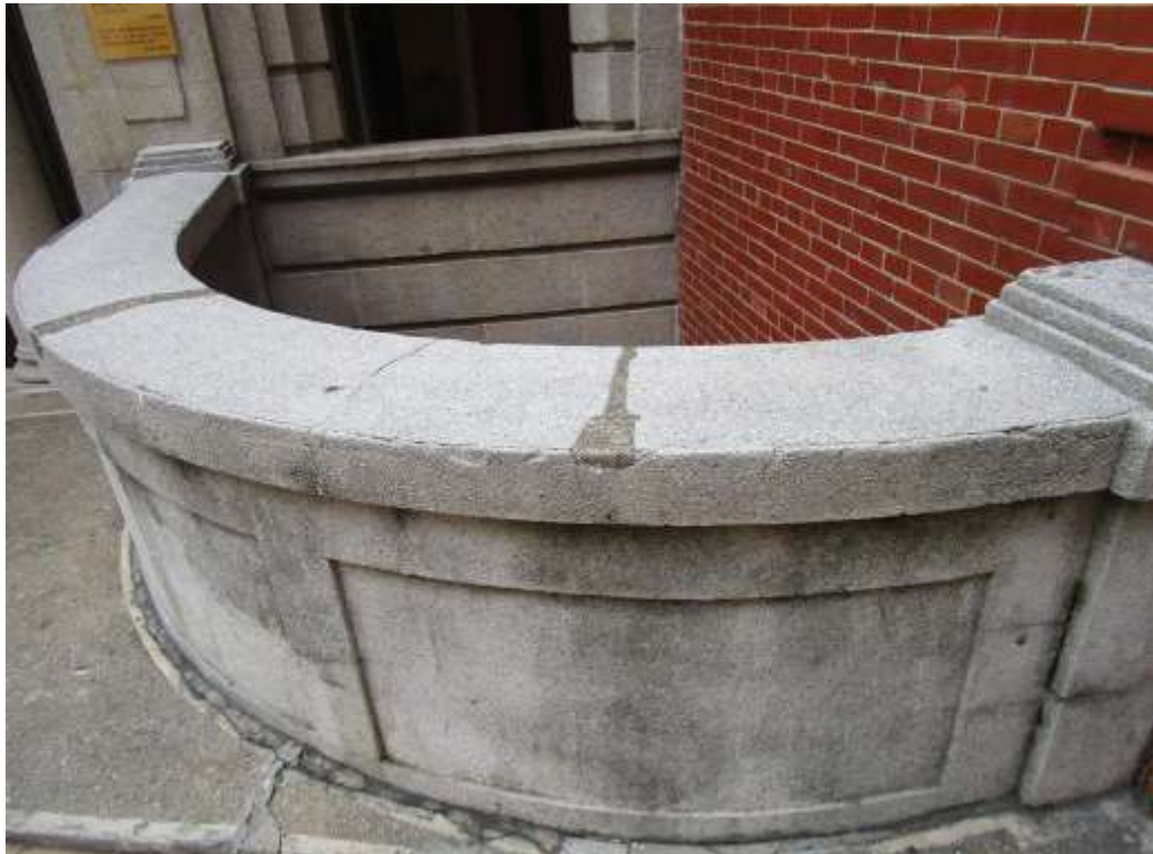
General View No. GV48 Description General view of parapet wall, east wing
