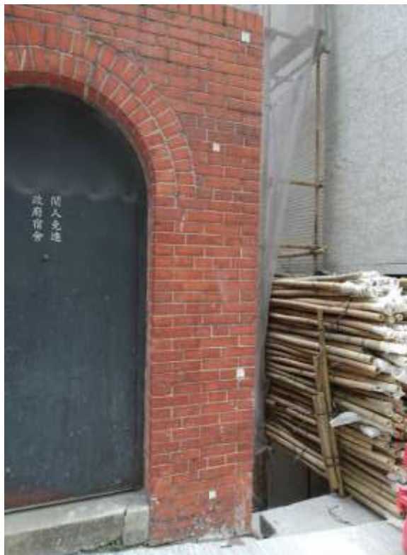
General View No. GV22 Description General view of survey mark on fence wall at northeast corner
