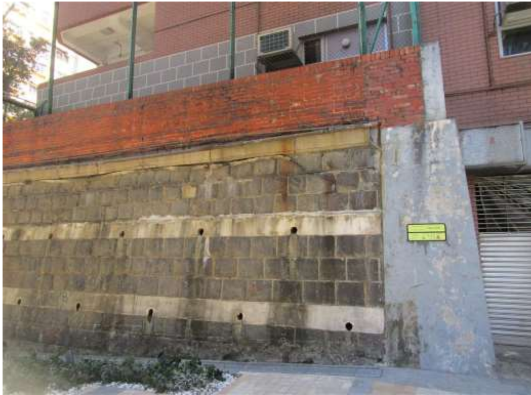
General View No. GV43 Description General view of west retaining wall under west wing
