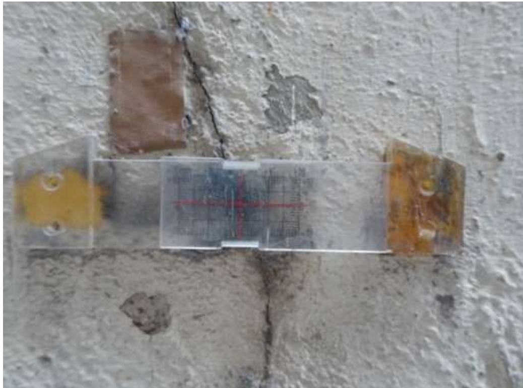
General View No. GV15 Description General view of tell-tale crack gauge on north retaining wall
