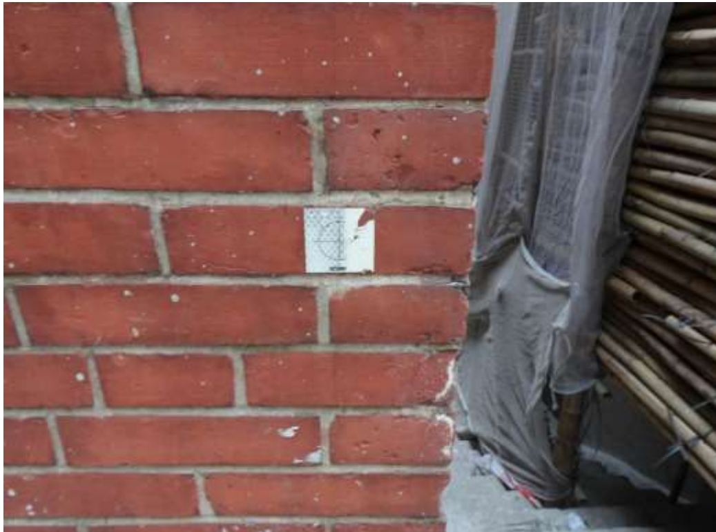
General View No. GV23 Description General view of survey mark on fence wall at northeast corner
