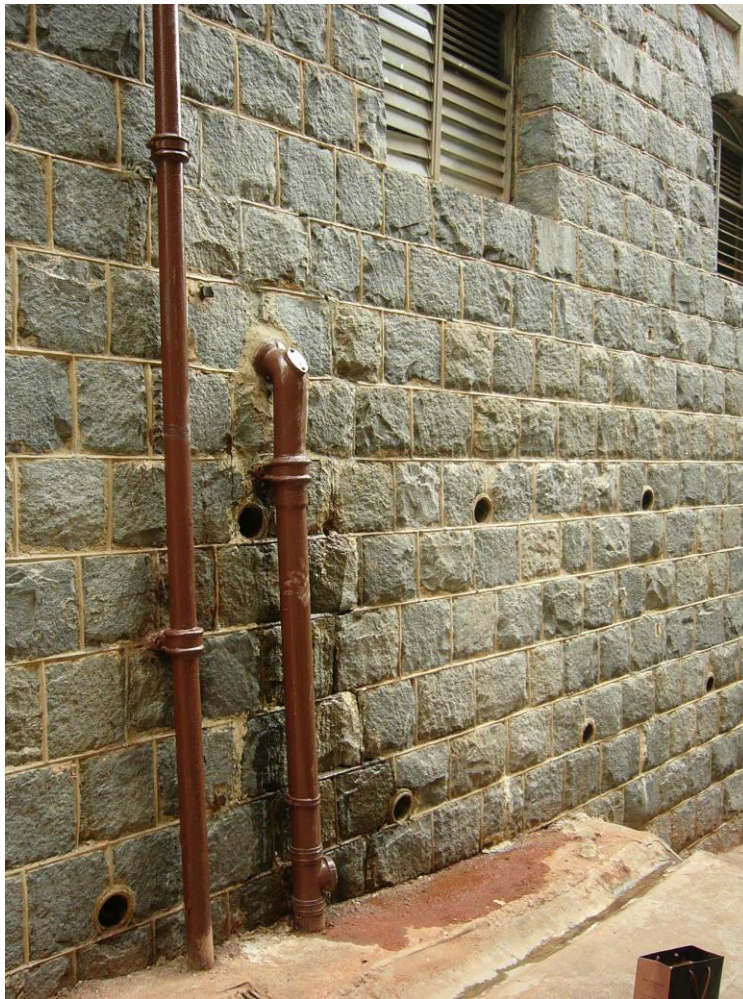
Plate 6: Water Seepage at the Middle Portion of the Masonry Wall
