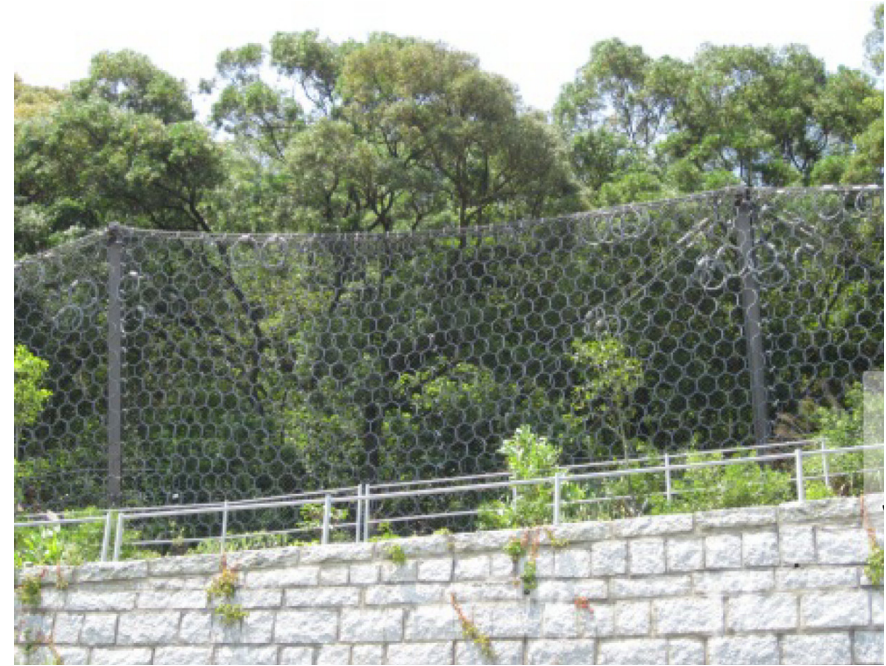
View of Flexible Barriers above Tung Chung Road
