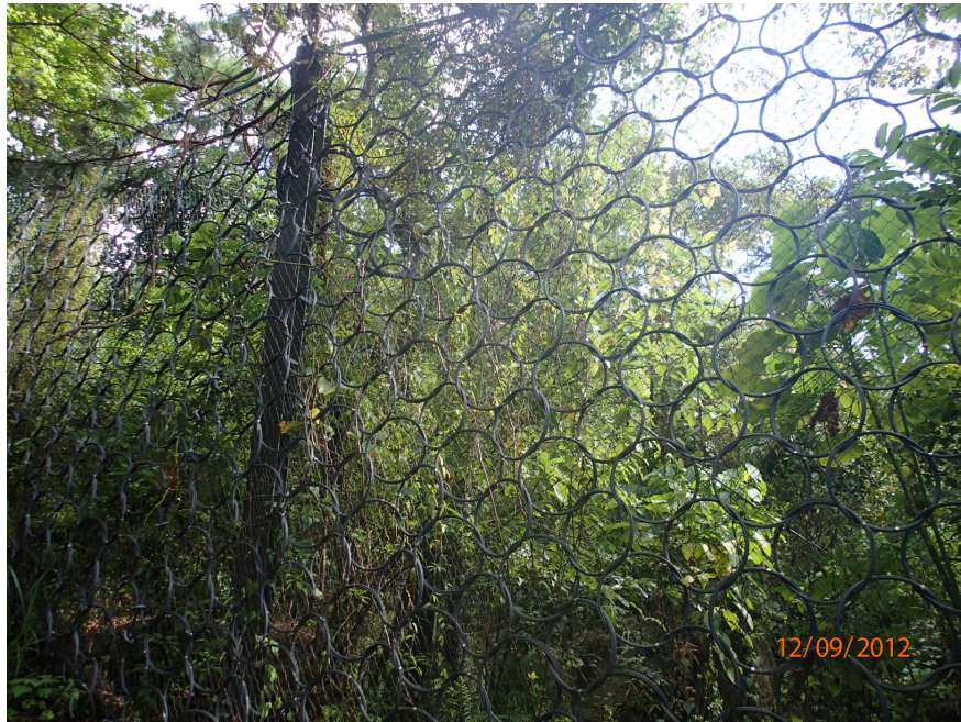
Close-up View of Flexible Barrier and Supporting Post
