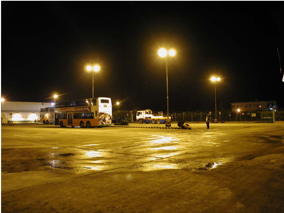
View showing the lighting system at TKO bus depot
