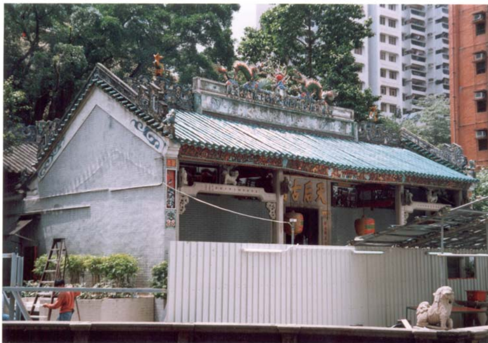
Photo 4 The temple roof has been sagging
