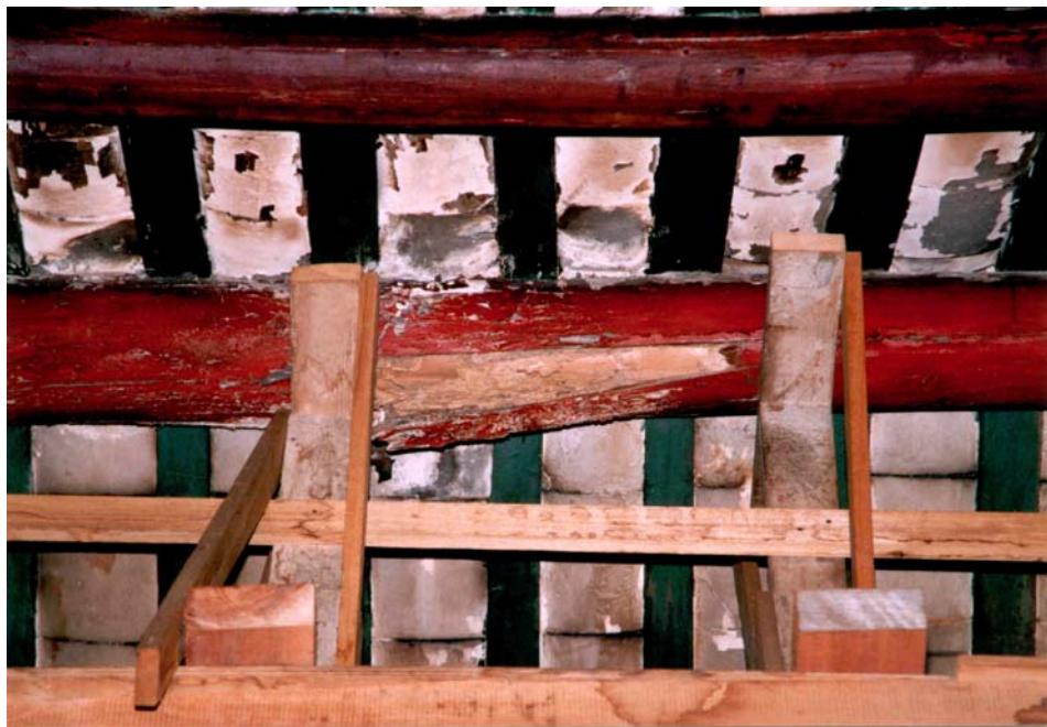
Photo 2 Termite infestation at the beams of the main hall of the temple
