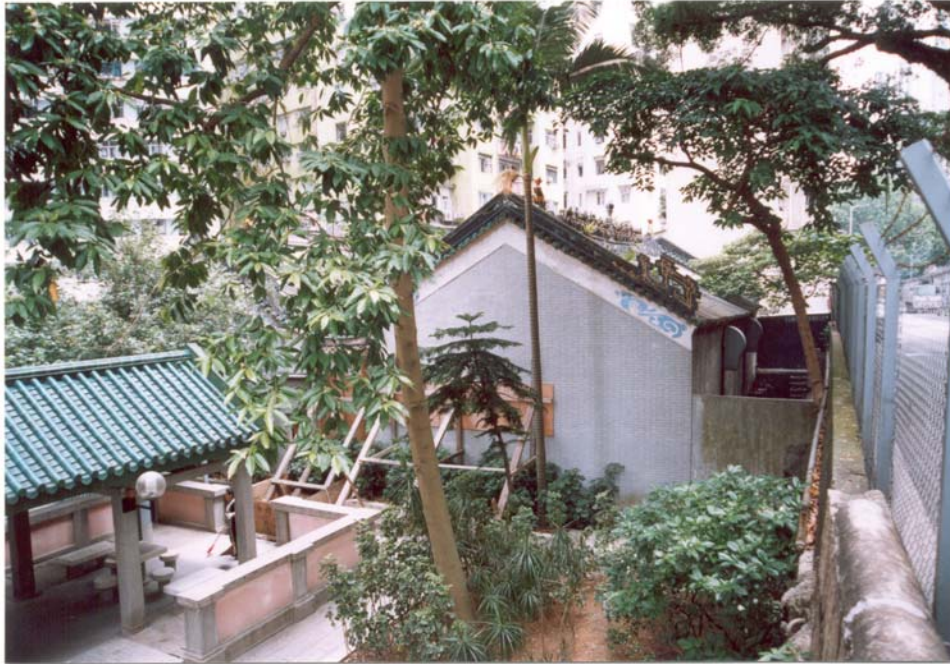
Photo 1 The Main flank wall has been bulged and is now being supported by temporary timber shoring
