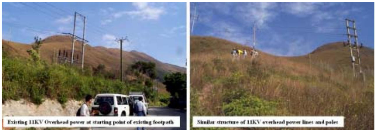
Figure 7: Example of overhead power line erected by CLP Power
