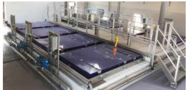
Eight SFK600 Salsnes Filters treating 2000 m 3 /h (12.6 MGD) at the Egå Wastewater Treatment Plant in Aarhus, Denmark.
