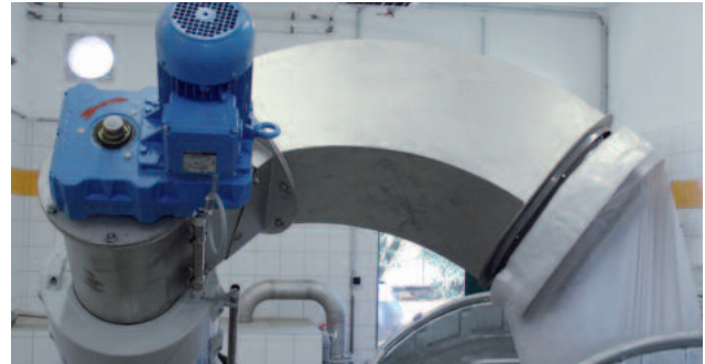
Individually adapted installation with lateral screenings discharge directly into a container
