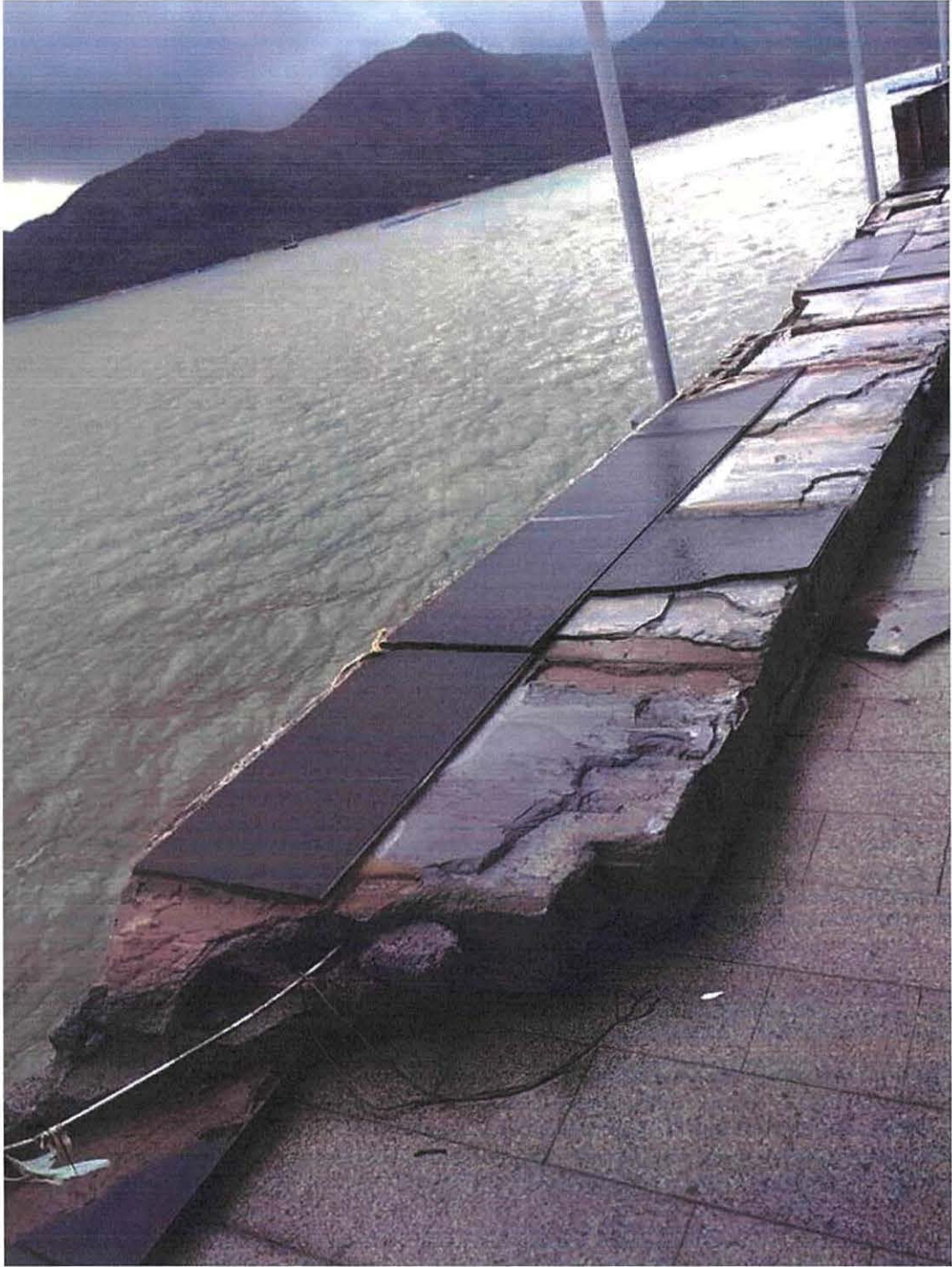
Damage in Sha Tau Kok Pier during Typhoon Mangkhut
