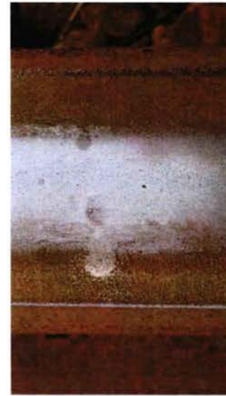
Running Surface of Far Rail WAL
