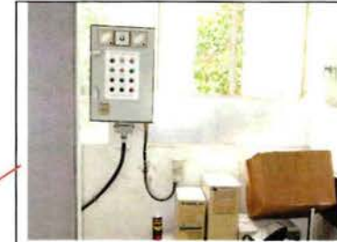
Item (1.2) Wall-mounted Control Panel
