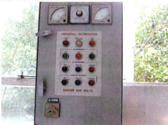
Photo 5 Wall-mounted control panel for the incinerator
