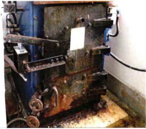
Photo 2 The incineration chamber door (top) and the bottom ash collection door (bottom) of the incinerator
