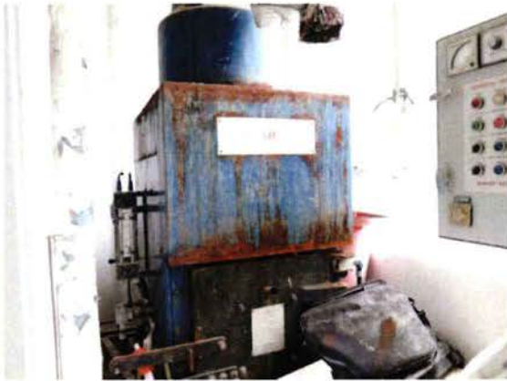
Photo 1 The incinerator at 5/F of UPB
