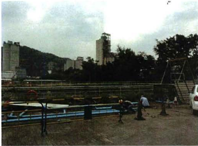
Photo 3: Temporary construction material storage area for Contractor at South of Lagoon No.1. The area is concrete paved.
