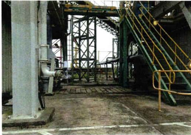
Photo 7: Existing ash silos along sea bank road west and the area is concrete paved.
