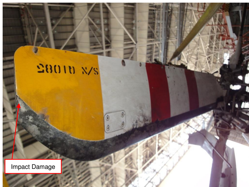
Figure 25 – Impact damage on Yellow blade
