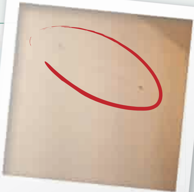
Fine cracks on wall
