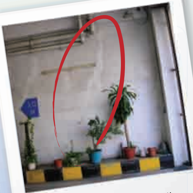
Cracks on partition wall
