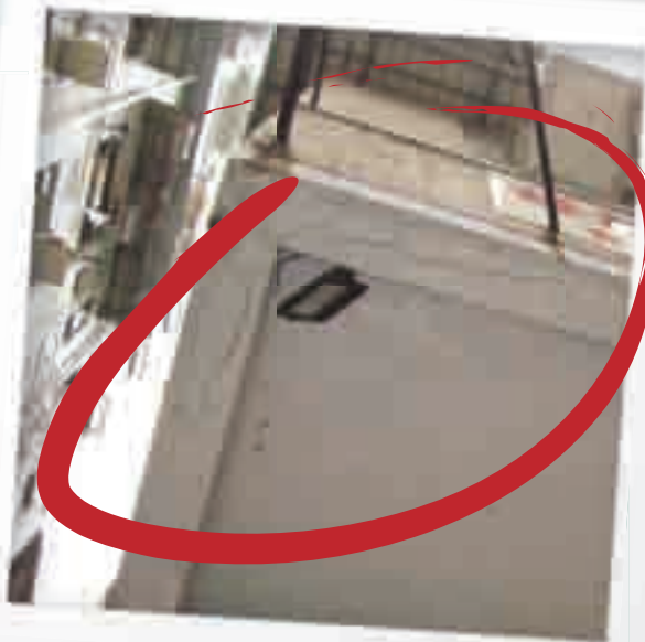
Cracks on the beam
