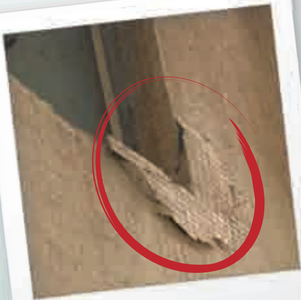
Bulging and loosening of wall tiles
