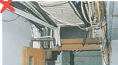
Services within staircase enclosure without proper protection
