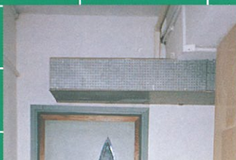
Cable and duct protection
